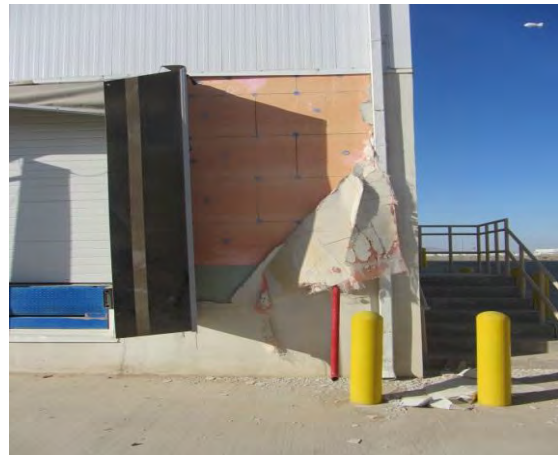
Photo 3 - Damaged Warehouse Siding
