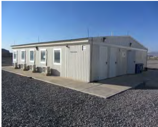
Photo 2 - Unshielded Heating/Cooling Units at Administration Building
