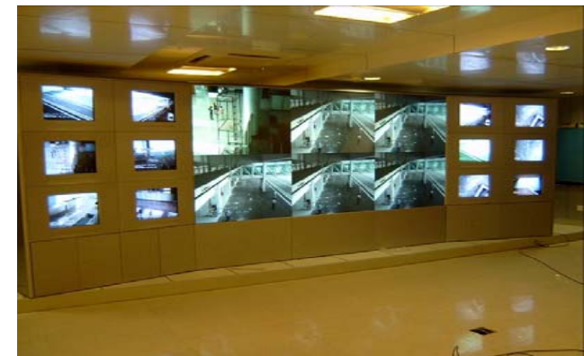
Multimedia Control Center in Customs at Baiyun Airport
