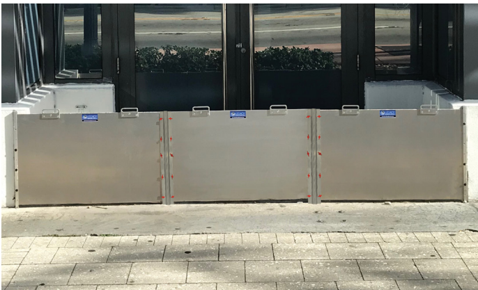
#5129MA mounted to front of hotel entrance.
