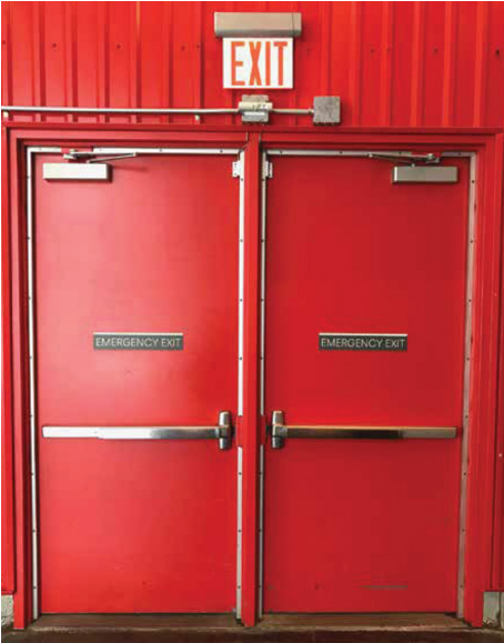
#5077 installed in conjunction with #5077SPB.
