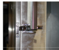
Door Latch Too High
