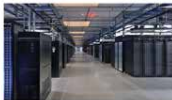
HOT AISLE CONTAINMENT
