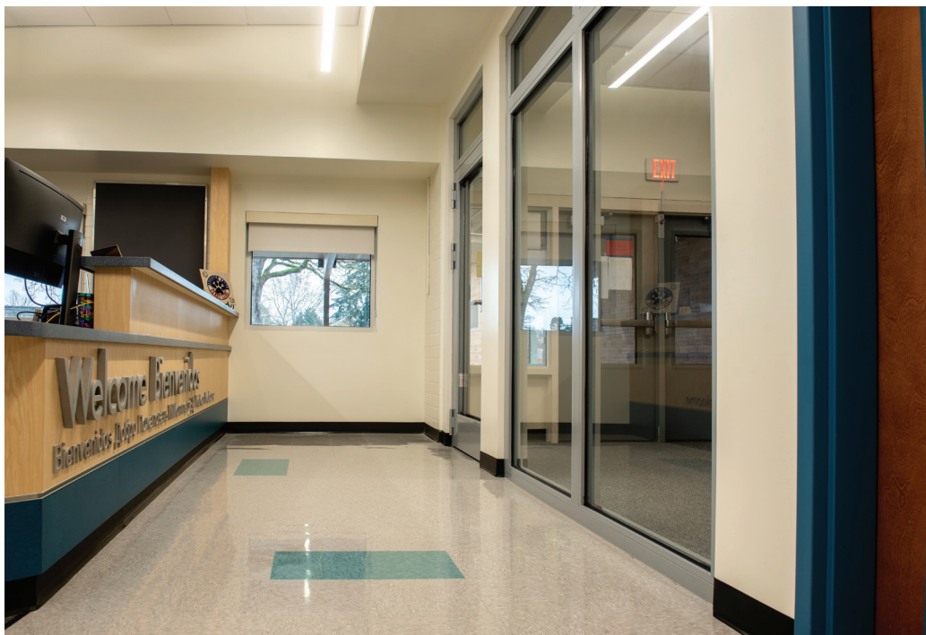
Straddling a central hallway and entry vestibule, the interior doors and windows of the main office needed to have a fire rating to satisfy code requirements.
