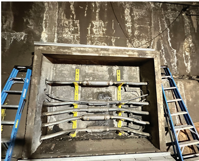
Electric cables inside junction box before access panel doors were installed.
