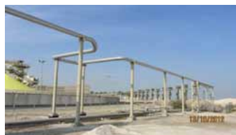
CO2 plant in Bapco
