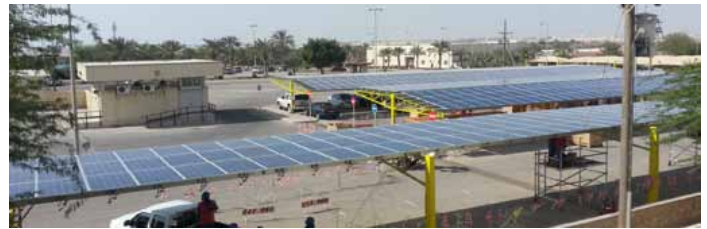
The $25 million Solar Project
