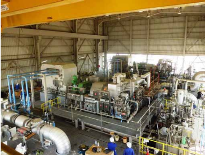
Interior shot of the STG plant
