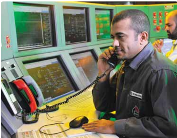
A control room at the Central Gas Dehydration Unit (CGDU) is part of the advanced gas production and transmission network.
