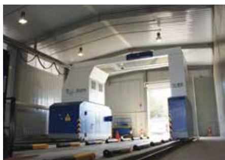
The inside of the Scanning Hall at Tlokweng Gate Border
