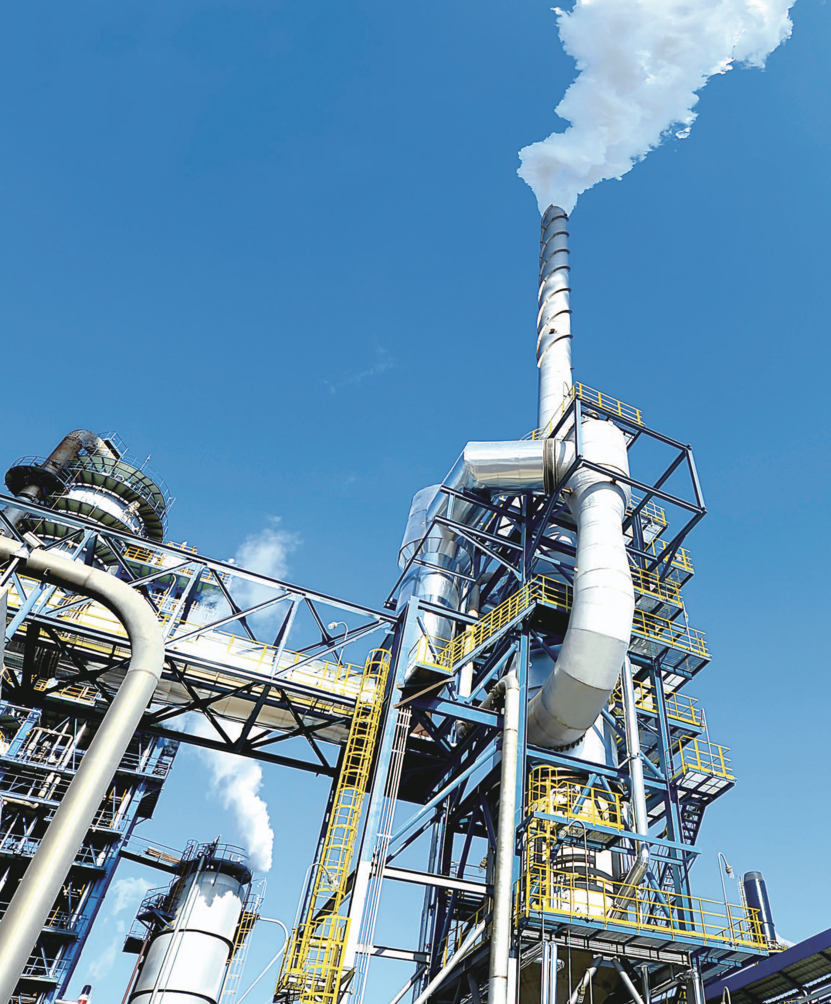
Flue gas purification facility at Jinxi Petrochemical
