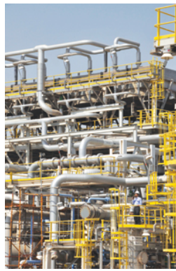
Bapco currently has two liquid LPG treating facilities
