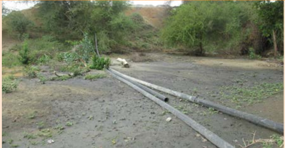
Tailings overflow from tailings dam
