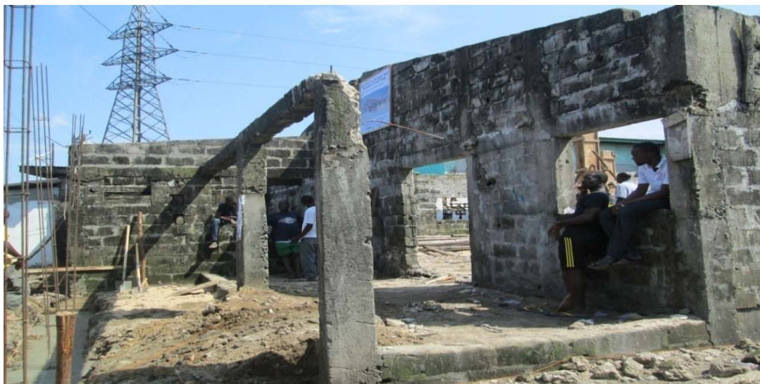
Abandoned West Point Town Hall Project for which US$40,000.00 was paid.
