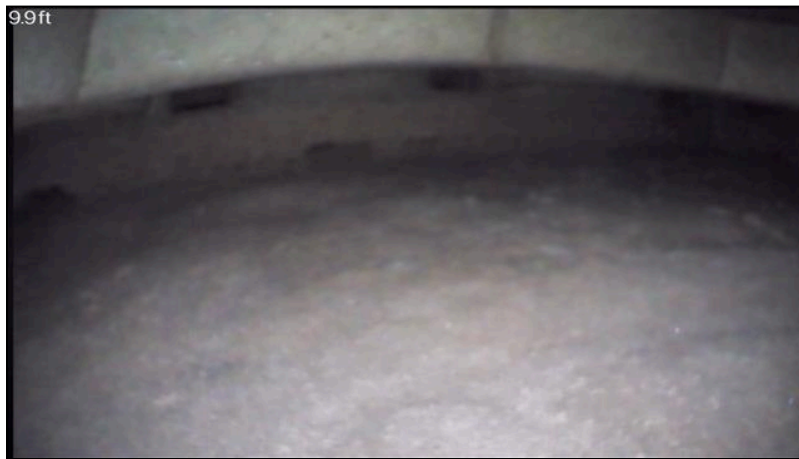
View inside chamber
