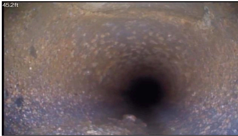
View of distribution line
