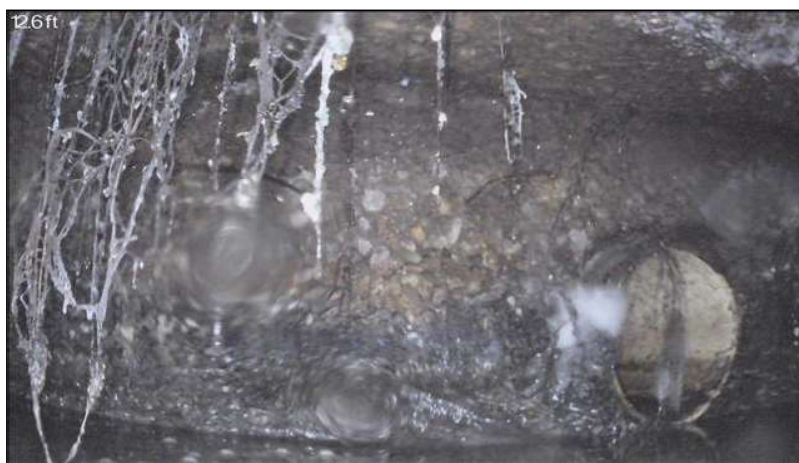
View inside D-Box
