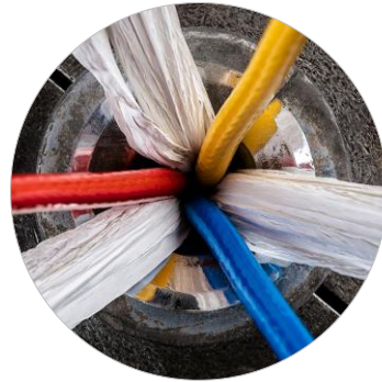
Fiber Optic Cables
