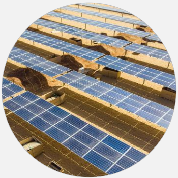
Solar Power Plants
