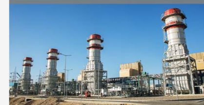
Attaqa Simple Cycle Power Plant Suez
