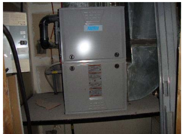
Furnace for second floor.
