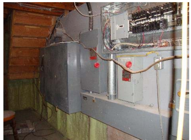
New electrical panel in basement.
