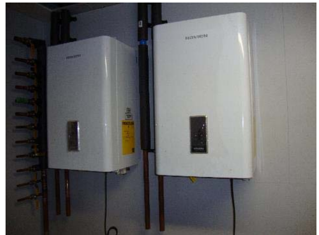
'On-demand' water heaters in basement mechanical room.
