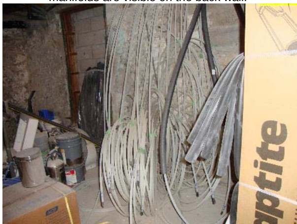
Piping for in-floor hot water heating system.
