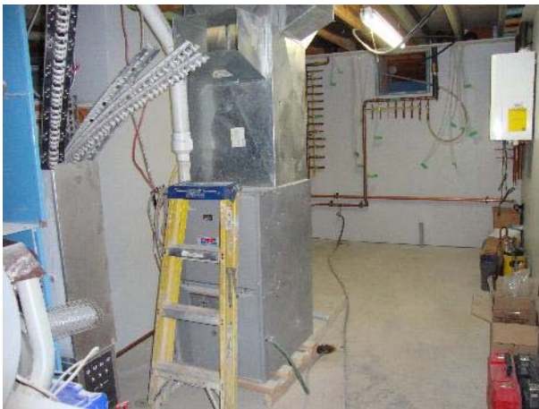
Mechanical room in basement with furnace. The 'on-demand' water heaters are visible on the right wall and the piping manifolds are visible on the back wall.
