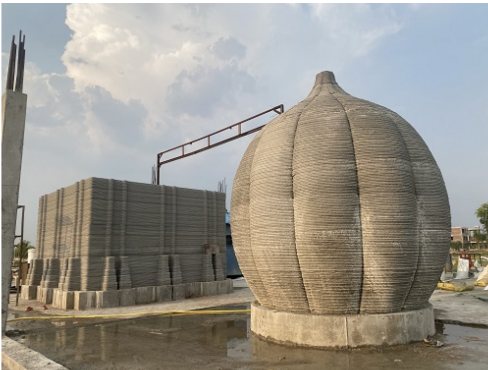
The 3D Printed Temple being built by Apsuja Infratech and Simpliforge Creations
