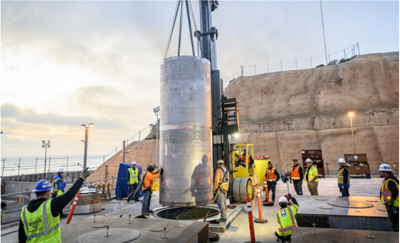
ISFSI aging management test canister and heater bank.
