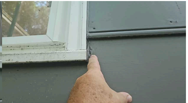
Rear right at garage window- siding moisture damage
