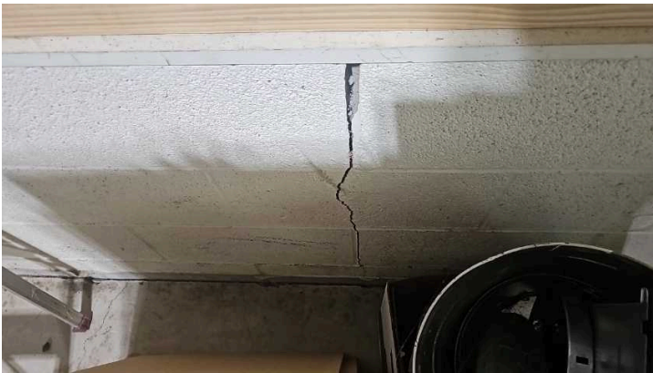
Unusual vertical crack in foundation
