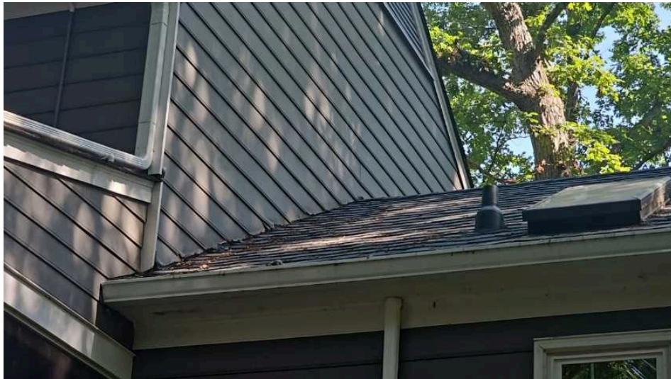
Left rear along roof- siding moisture damage
