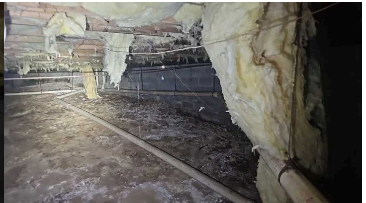
Stringy insulation indicates long term moisture problem
