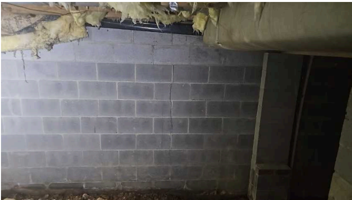
Unusual cracking in foundation on far left
