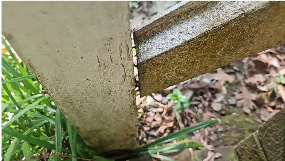
Separation in railing
