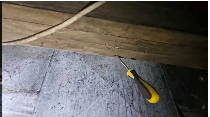
Probing rot on floor structure
