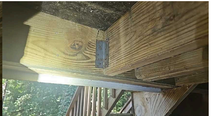
Metal framing brackets has rusty nails
