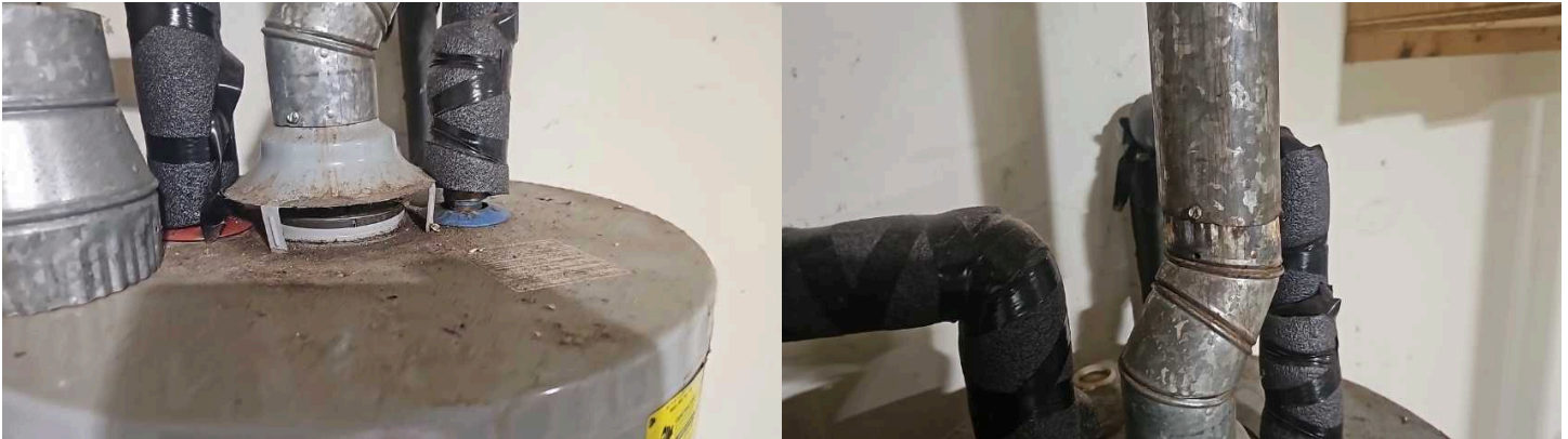
Flue pipe not secured properly
