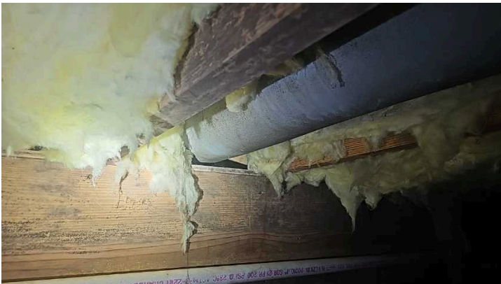
Fungal like growth on floor structure
