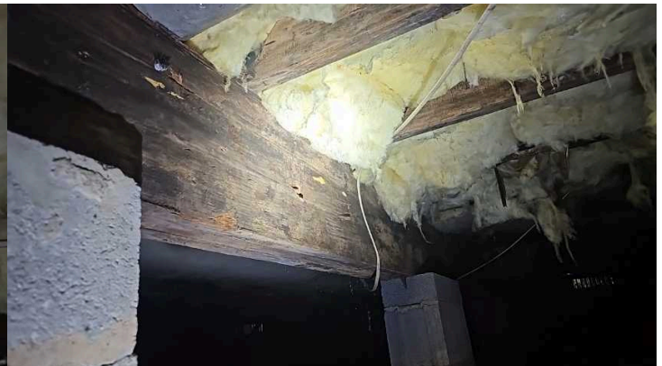
Black fungal like growth and rot on floor structure
