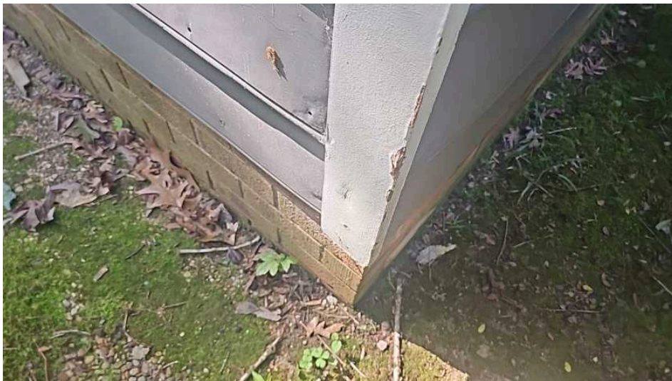
Front right corner trim damaged
