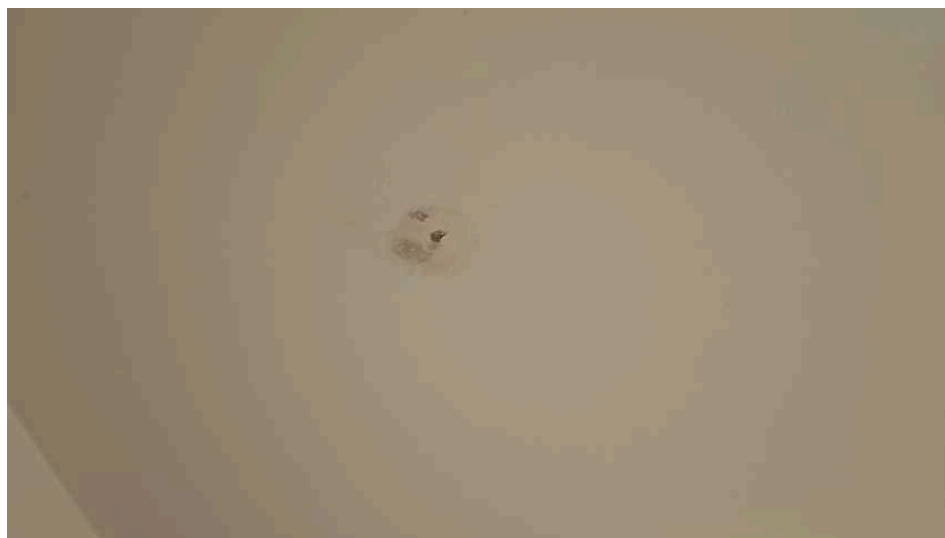
Stain in Upper rear middle bedroom...old
