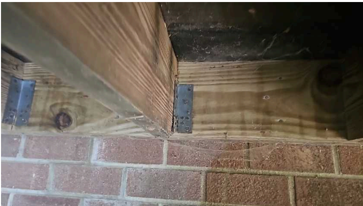
Metal framing brackets has rusty nails
