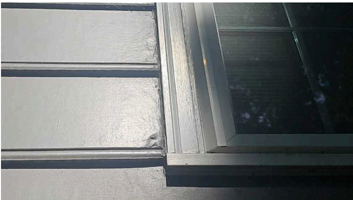
Left at window- siding moisture damage
