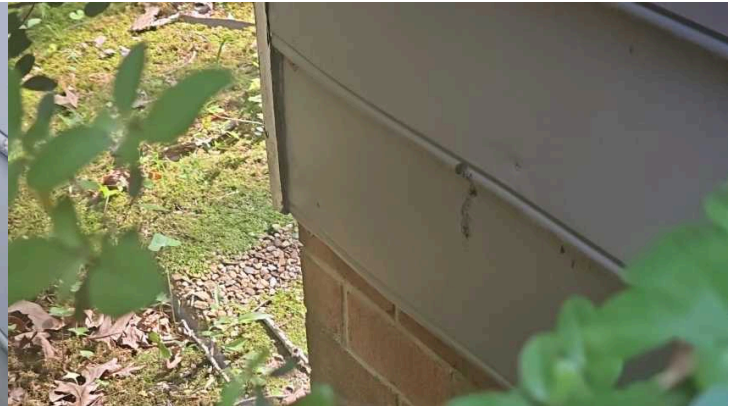
Right front behind overgrown shrub- siding moisture damage
