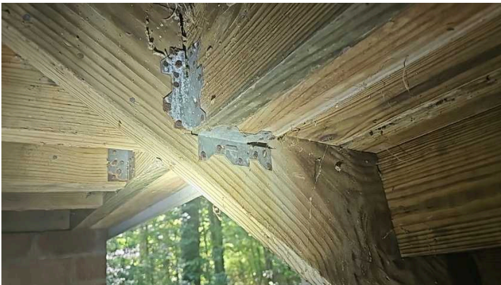
Metal framing brackets has rusty nails
