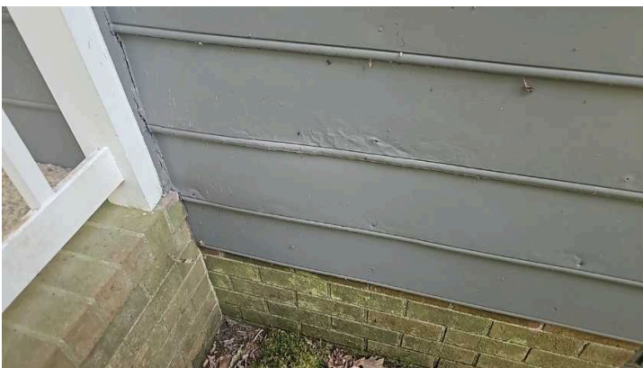
Front near porch- siding moisture damage
