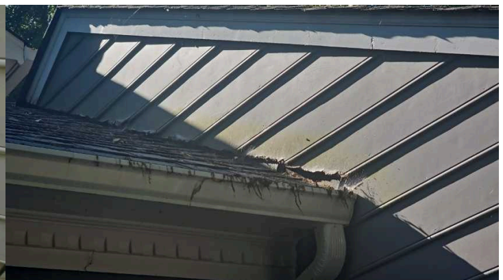
Right along roof - siding moisture damage
