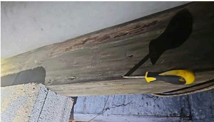
Probing rot on floor structure
