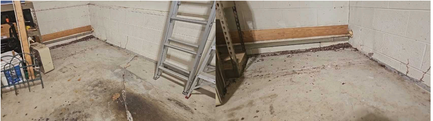
Unusual horizontal crack in foundation
