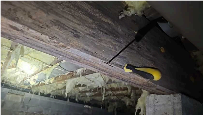
Black fungal like growth and rot on floor structure
