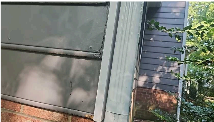
Left front corner - siding moisture damage
