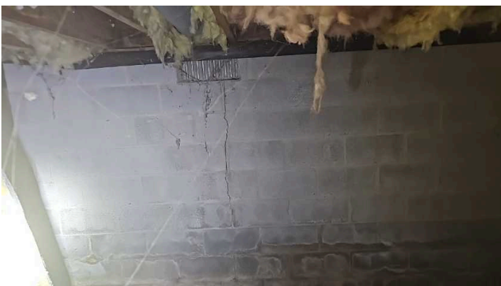
Unusual cracking in foundation on far left
