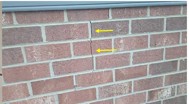
Cracking in brick on rear exterior of garage
