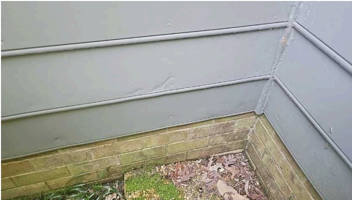
Right front inside corner- siding moisture damage
