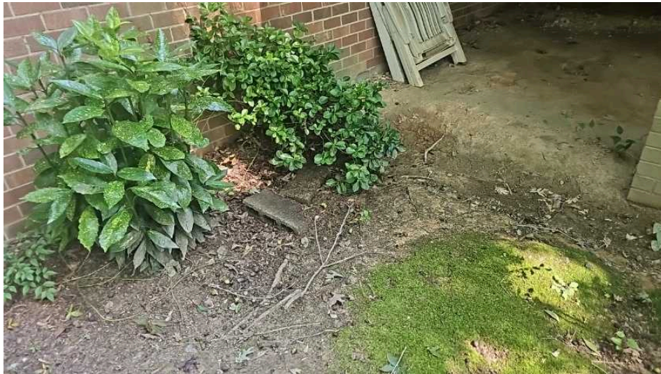
Sunken area on rear near porch
