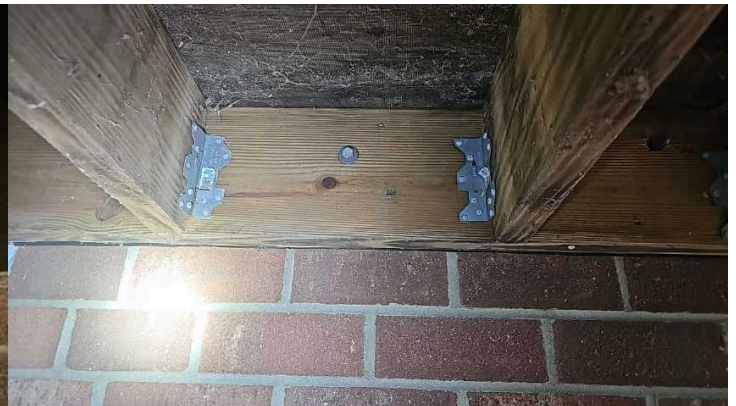
Some nails are not rusty
