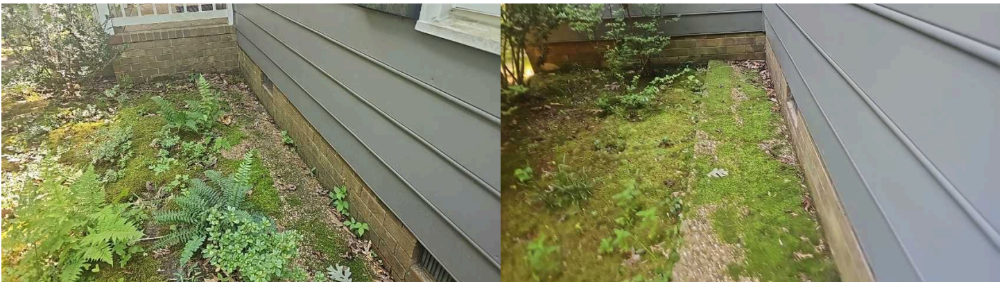
Concrete apron is rotated and sloped wrong direction
