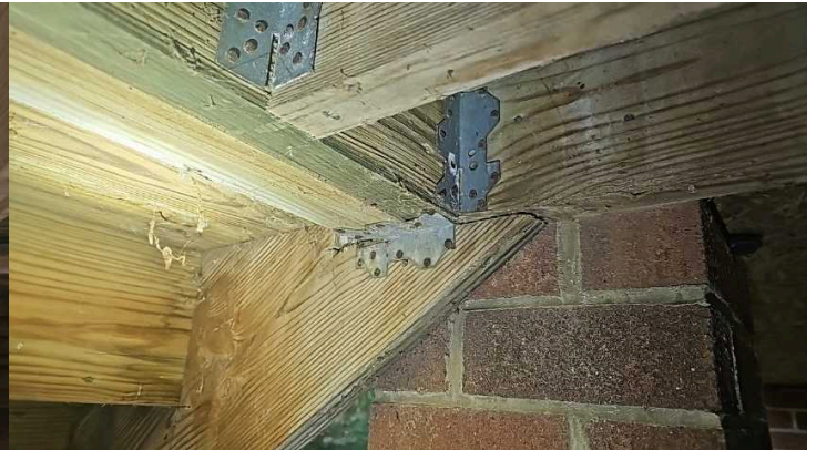
Metal framing brackets has rusty nails
