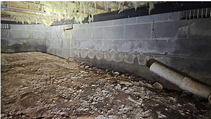
Wet foundation adjacent to the concrete apron on front
