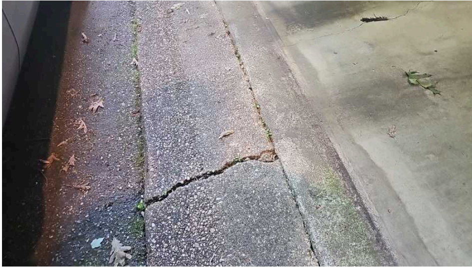
Concrete apron at garage door is cracked
