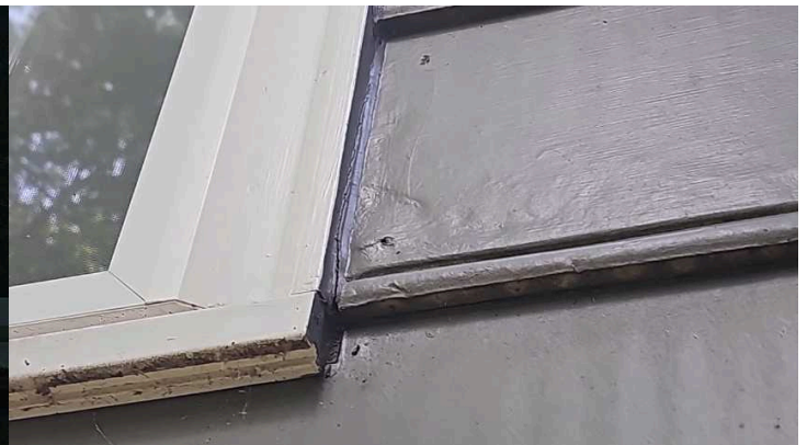
Left at window - siding moisture damage
