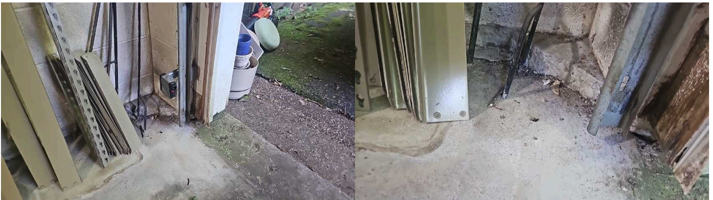
Concrete settled at least 3"
