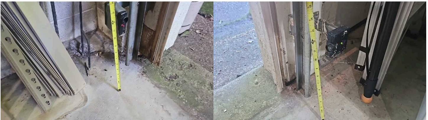
Photo sensor measuring 12" off floor on side where floor has settled
