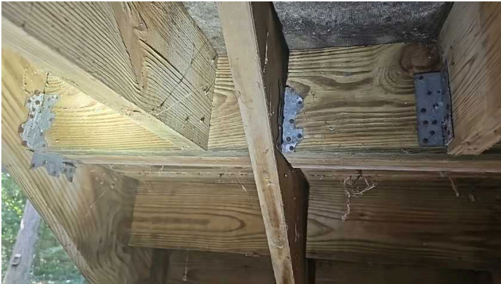
Metal framing brackets has rusty nails
