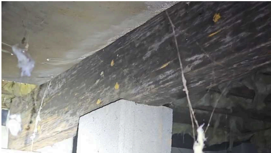
Black fungal like growth and rot floor structure
