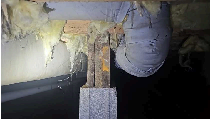
Fungal like growth on floor structure
