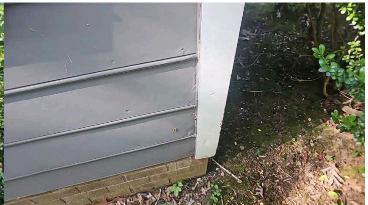
Front right corner - siding moisture damage
