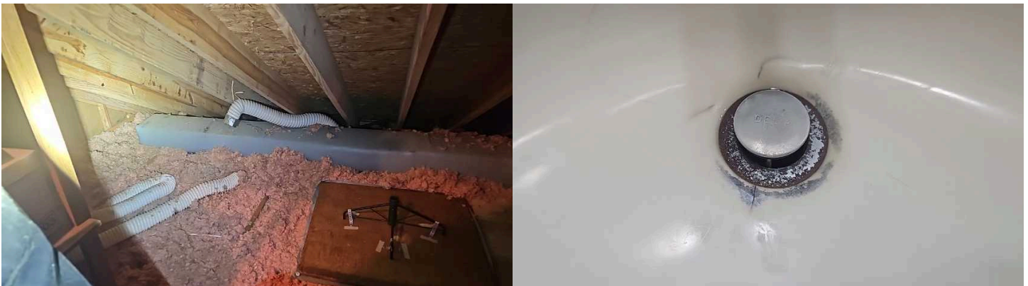
Exhaust duct disconnected in attic
