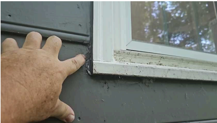
Rear right at garage window- siding moisture damage
