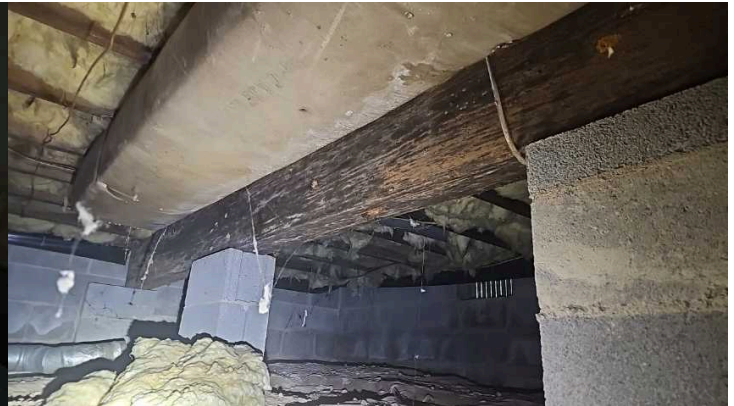
Black fungal like growth and rot floor structure
