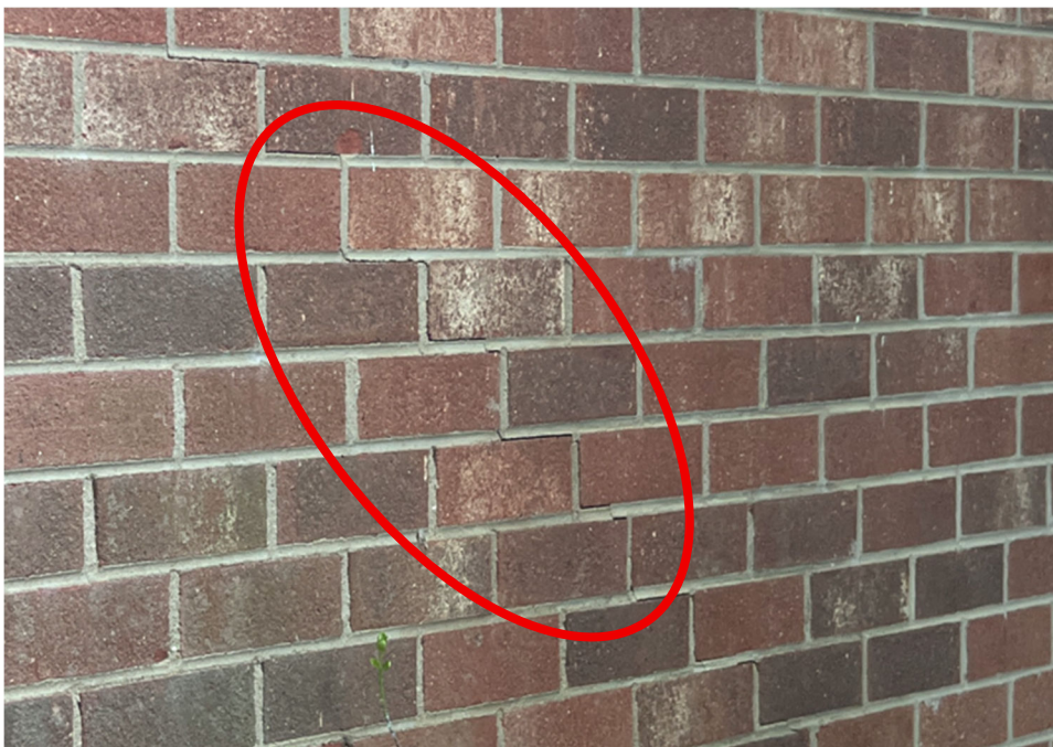
Stair step settlement cracks.
