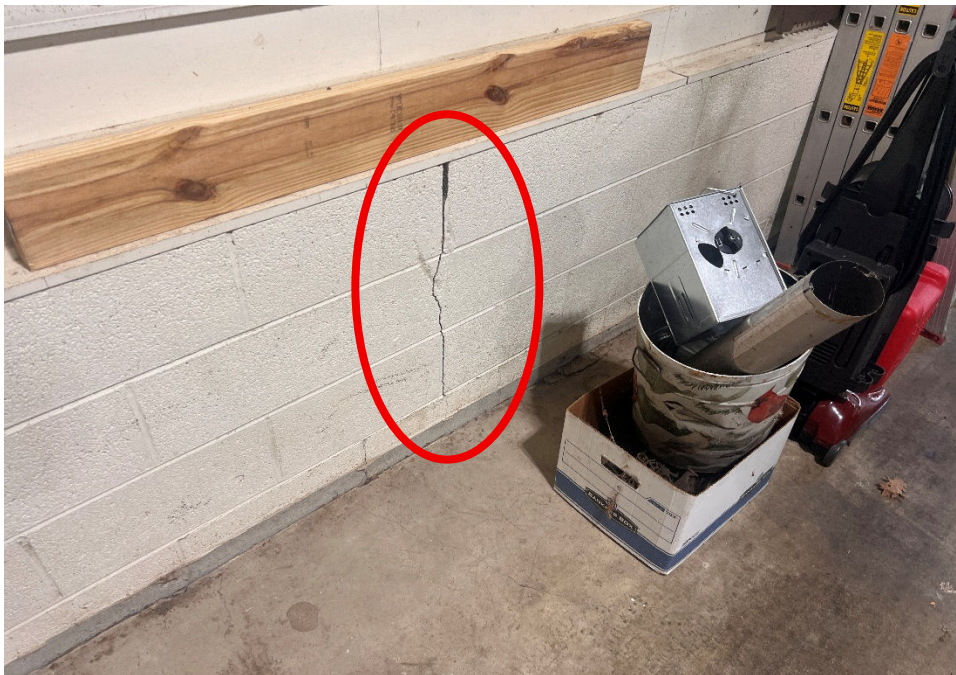
Cracks in the CMU wall in the garage.
