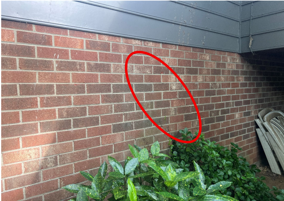
Cracks in the brick sheathing behind the garage.
