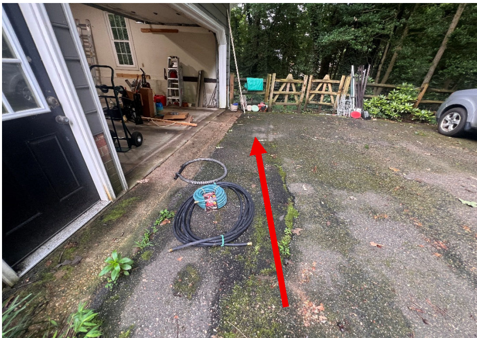
Water flows down the asphalt driveway and arrives at the garage.
