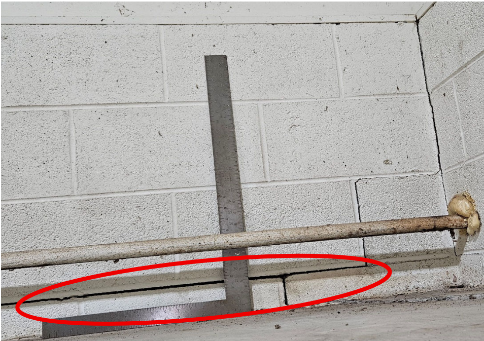
Horizontal and stair step cracks in the garage.
