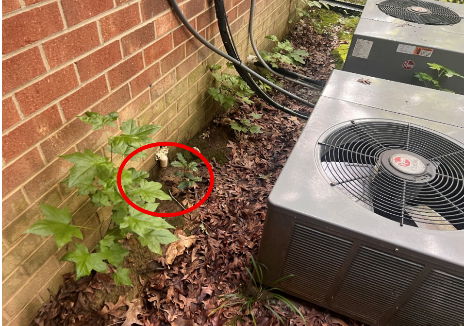
The HVAC condensate line is discharging too close to the homes foundation.
