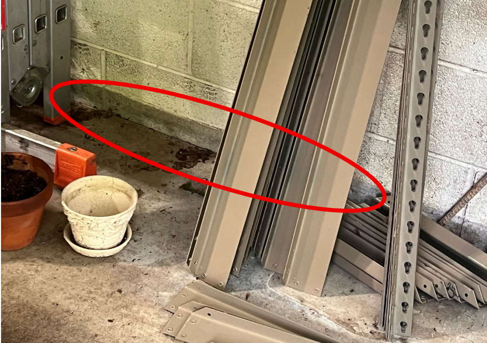
The concrete slab has sunk approximately 4 inches.
