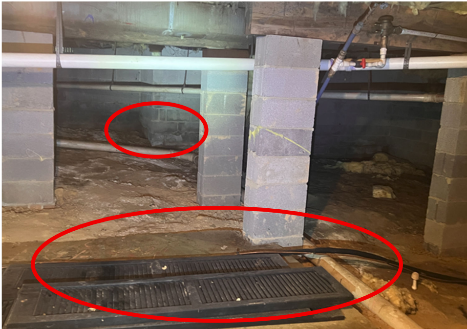
Conditions under the home are damp and wet in places. Efflorescence stains are prevalent.
