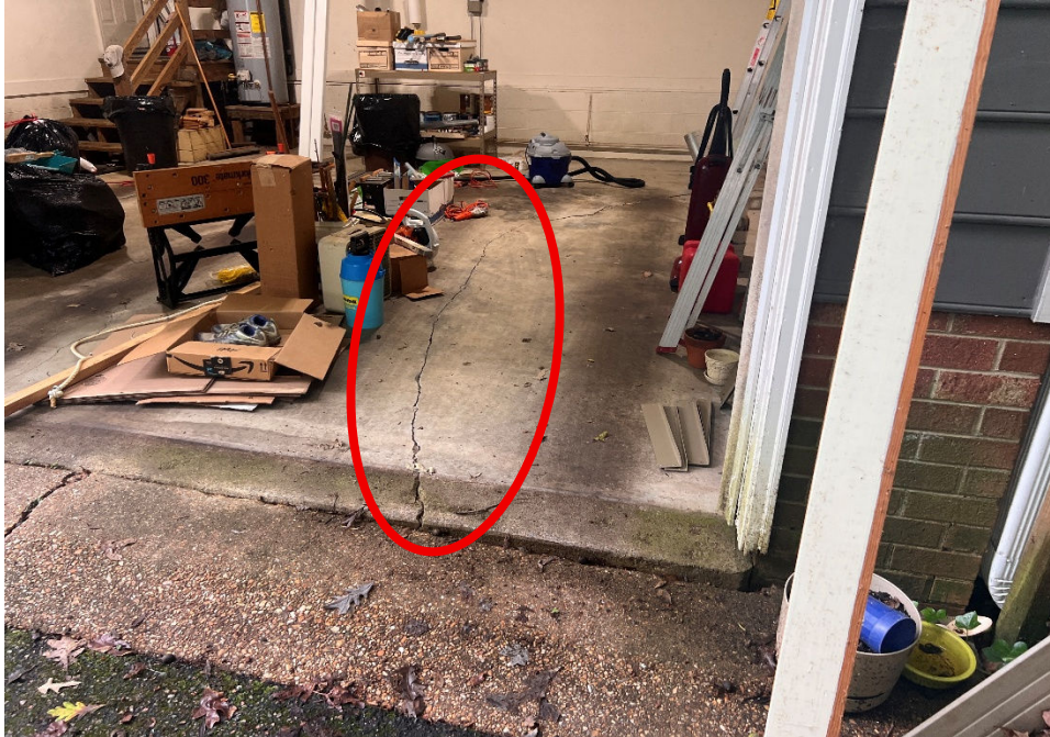
The garage slab has cracked in several places.
