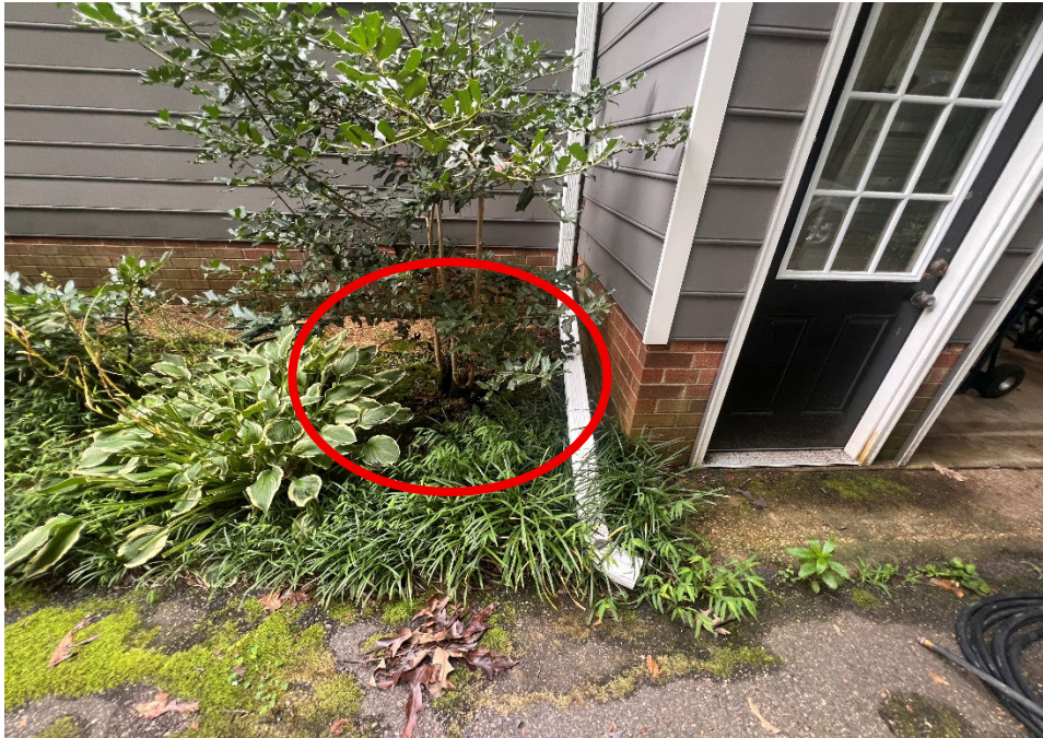
Water ponded here for many years before gutters were added. This downspout has been piped away from the foundation, to the front of the garage.
