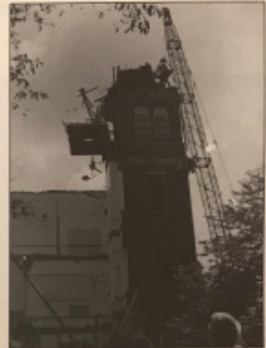
The last Old Main tower comes down in 1958. The niche visible on the third floor is in the remaining wall of the Union Literary Society Hall.
