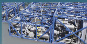
Skid Mounted Frac Pumps
