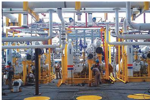
The fully automated MGS is designed to handle production of multiple wells. (Source: Leistriz)
