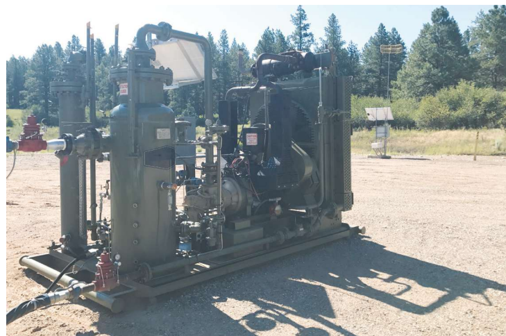
A Flogistix rotary screw compressor is on location performing wellhead drawdown. (Source: Flogistix)
