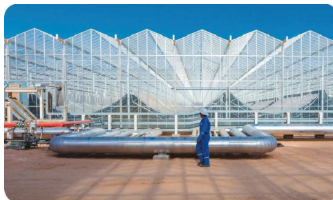
GlassPoint Solar has developed a solar steam production facility in Oman for use in EOR efforts. (Source: GlassPoint Solar)
