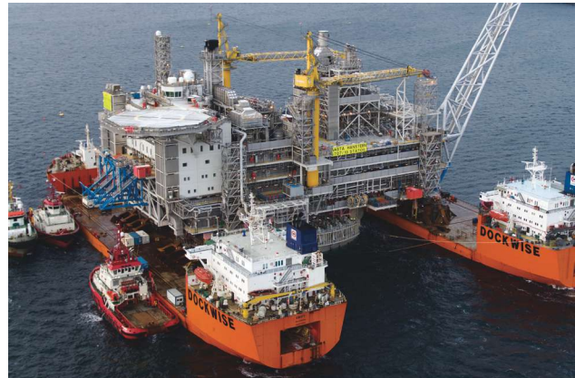
The Aasta Hansteen topside is balanced across the hulls of two S-class vessels as it is mated to the spar offshore Norway. (Photo by Espen Rønnevik/Worldcam, courtesy of Statoil)
