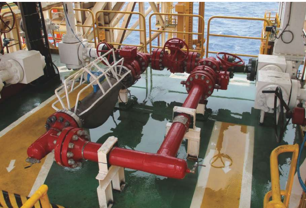
The Coriolis meter (in gray) monitors fluid flow of the MPD system, enabling accurate hydraulic modeling for real-time pressure control. (Source: Halliburton)
