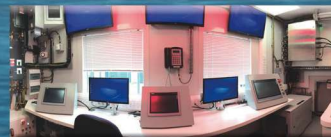
Automated Frac Controls & Master Fracq Data Acquisition Systems
