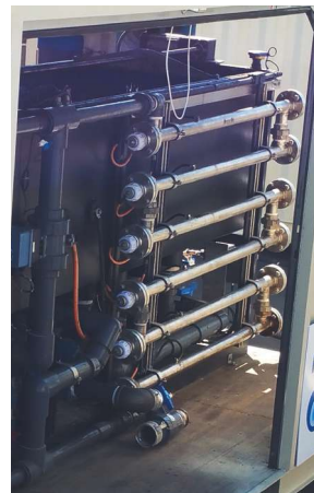
The ECOPOD system is operating in a Kern County oil field, cleaning 340 bbl/d of oilfield wastewater and salvaging it for agricultural irrigation. (Source: OriginClear Inc.)
