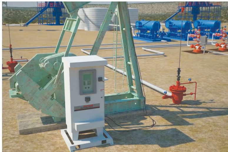
The equipment components required on sites can include lease automatic transfer units, compressors, pumps and more, with all requiring new reliable multiwell pad solutions to manage and control operations. (Source: Rockwell Automation)
