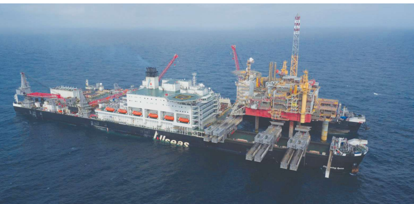
The Pioneering Spirit straddles its twin bows around the Yme platform before securing the structure, cutting the jackup facility’s steel legs and lifting the 13,500-tonne topsides. (Source: Allseas)
