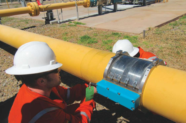
Clamp-on flowmeters enable monitoring of production in real time. (Source: Expro)
