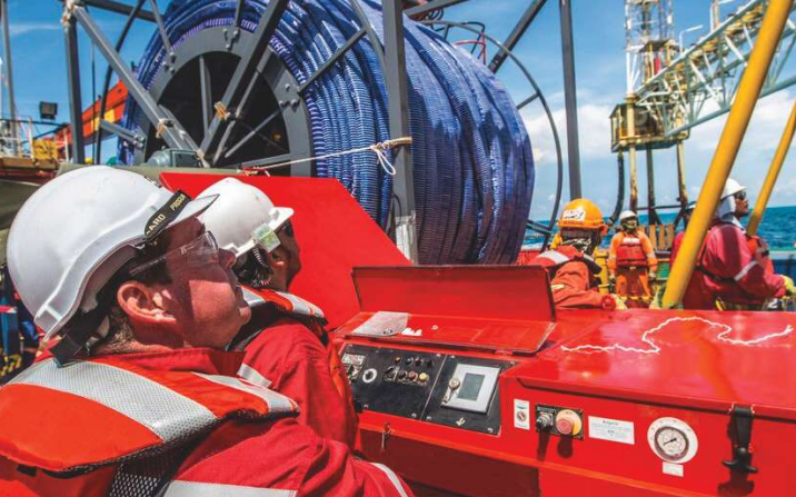
A shipboard crew deploys the IFL system at the PCSB Field. (Source: Anticorrosion Protective Systems LLC)
