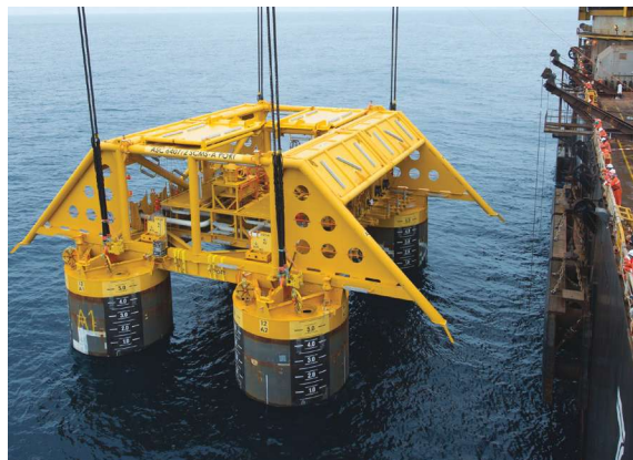
One of the subsea templates being installed on Statoil's Åsgard Field offshore Norway is shown. As subsea operations further extend into more remote and challenging environments, the need for alternatives to water-based subsea control fluids will increase. (Source: Statoil)
