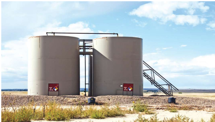
SCADA systems can alert operators to situations like when a tank is nearing capacity. (Source: rCarner/Shutterstock.com)
