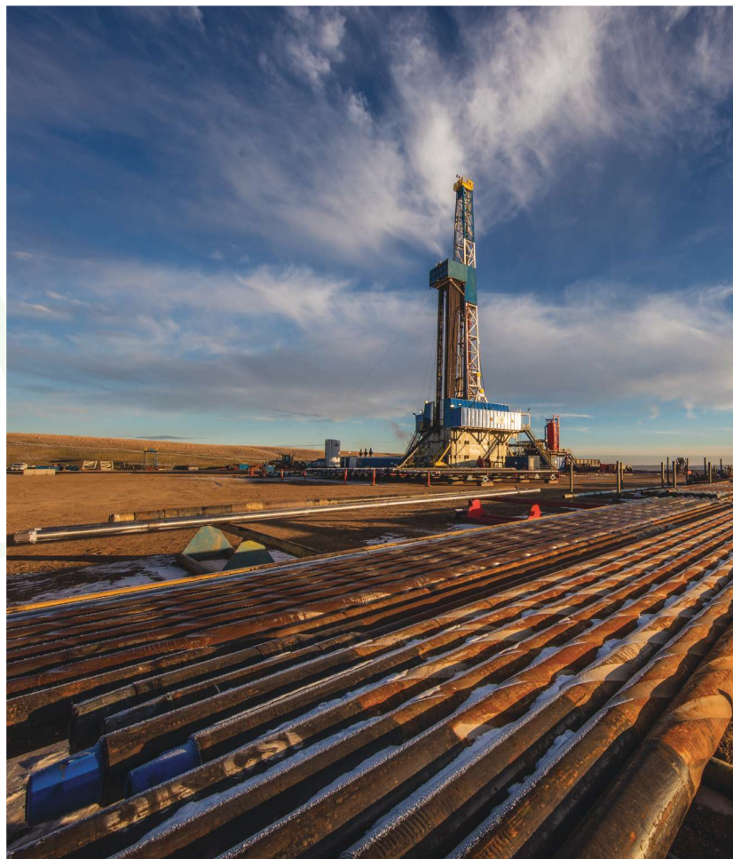
Through Lean manufacturing processes, Hess is continuing to increase efficiency and in turn bring down drilling costs in the Bakken. Pictured is the Nabors B06 Rig drilling a Hess well in December 2015 just south of Tioga, N.D. (Source: Hess Corp.)
