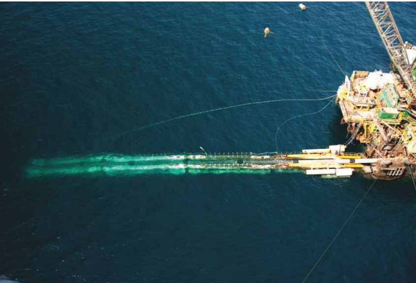
Pipelaying takes place offshore Qatar connecting the North Field to the Qatar-gas LNG facility at Ras Laffan as part of Qatar Petroleum and Shell's Qatargas 4 LNG project. (Source: Shell)
