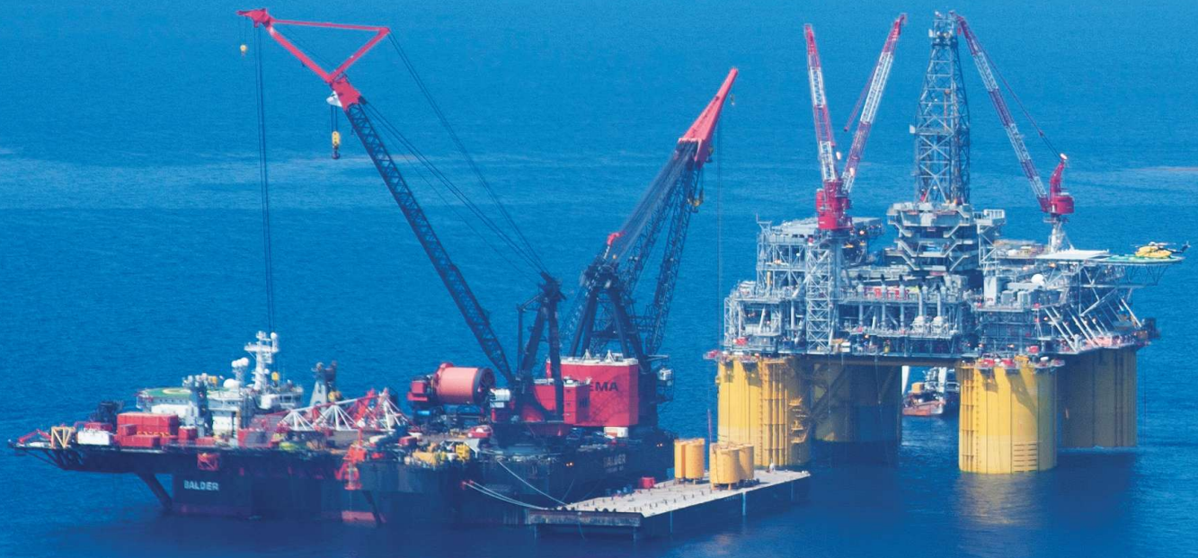
Heerema's Baldur deepwater construction vessel at work installing Shell's new Olympus platform next to Shell's Mars platform in the GoM. (Source: Shell)
