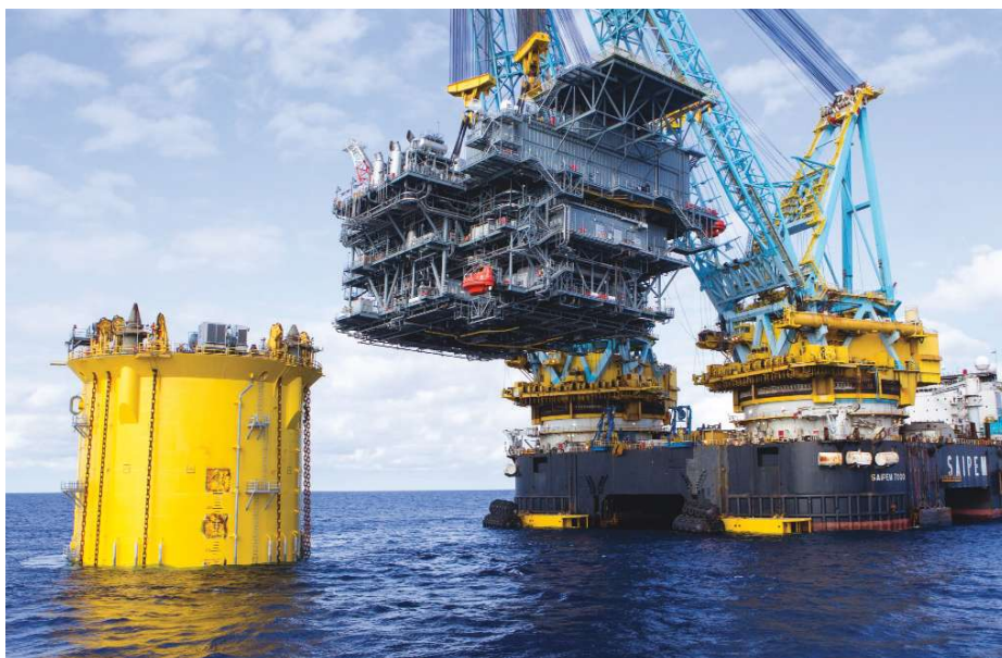
The Saipem 7000 heavy lift vessel installs the three-deck topsides in a single lift onto the Tubular Bells spar hull. The completed topsides weighed about 7,000 mt. (Source: Hess)
