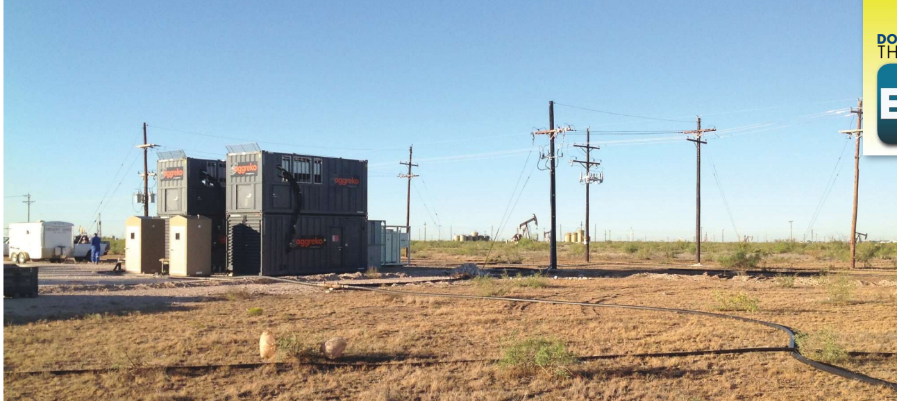
A stranded gas temporary power application is seen operating in West Texas. (Source: Aggreko)
