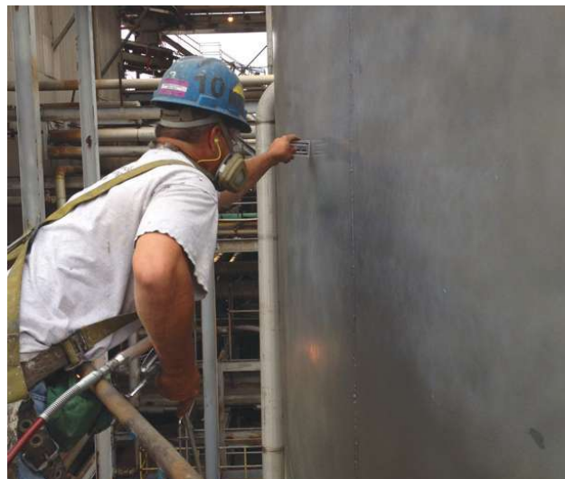
A technician measures the thickness of the nanomaterial on a tank wall. (Source: Industrial Nanotech Inc.)
