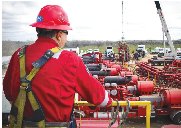
In a Northeast U.S. shale play, Weatherford returns to an unconventional well that has been determined to be a good candidate for a refracturing operation. (Source: Weatherford)
