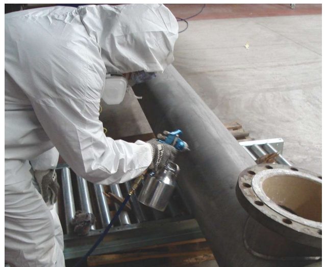
The Nansulate coating is sprayed on a steam pipe. (Source: Industrial Nanotech Inc.)
