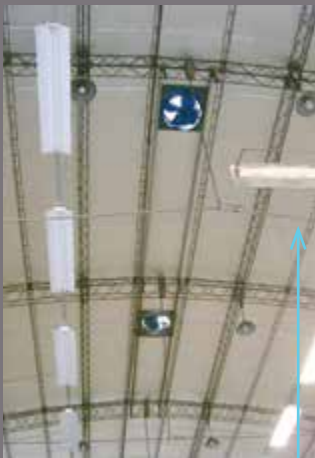
Reflective insulation, like this white-faced product, also can help illuminate structures.
