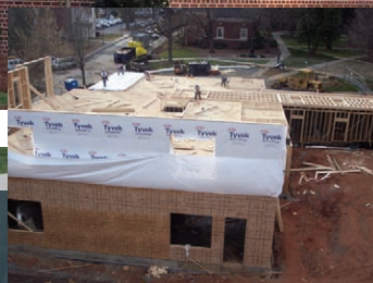
2007 Hayes Building, connected to Burris Hall, was under construction in 2006 (right) Hayes Building was complete in 2007 (above).
