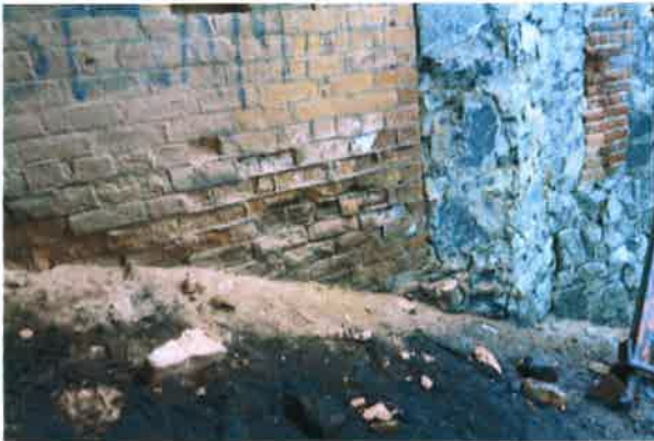
Brick delamination in the Chimney-Flume transition.
