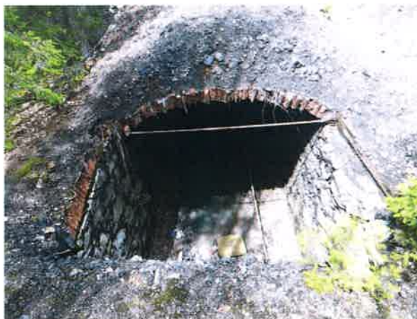
Flume collapsed section.
