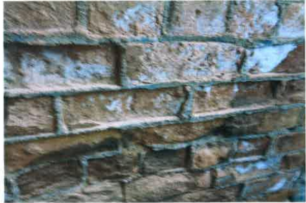
Detail of the brick delamination.
