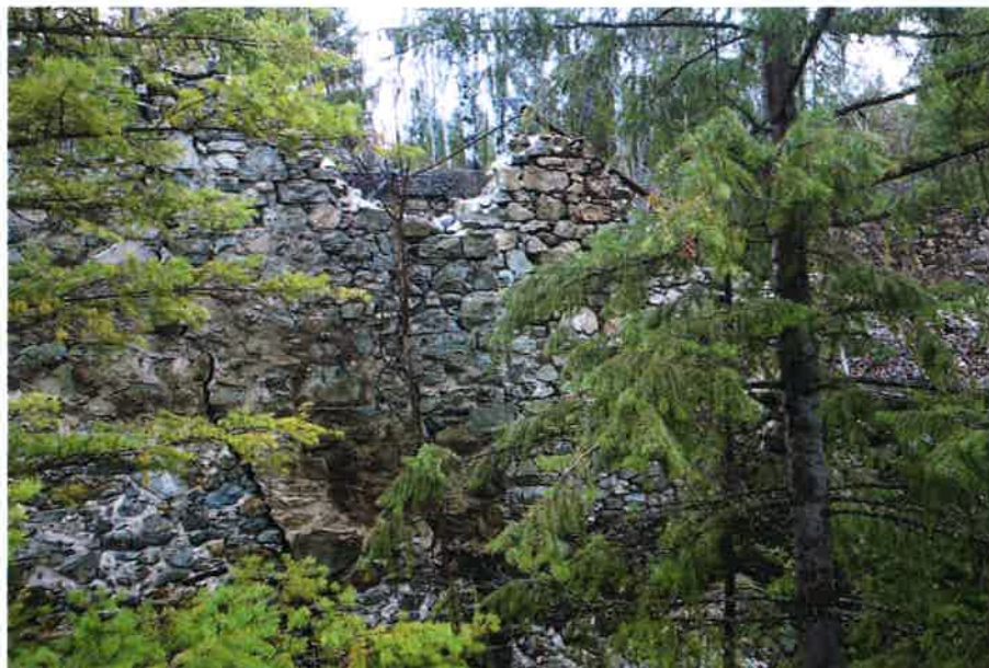
Crack along the masonry wall.
