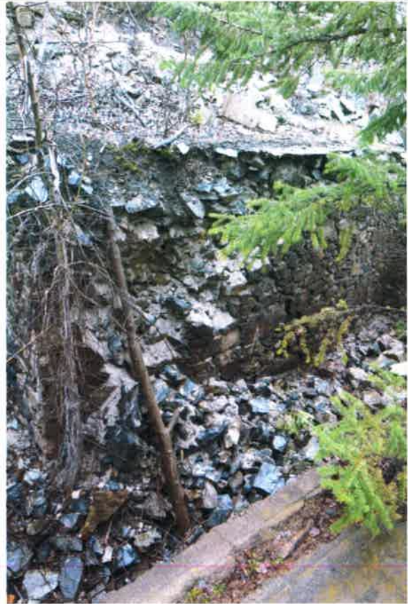
Washed mortar and salt deposits on masonry wall.
