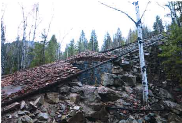
Partially collapsed masonry roof of the Flume.
