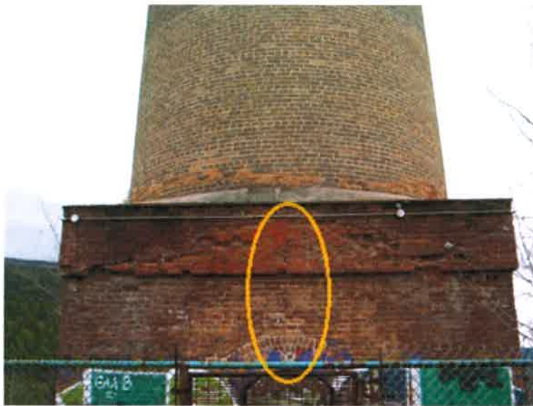
Figure 3 - Vertical Crack in Stack Base
