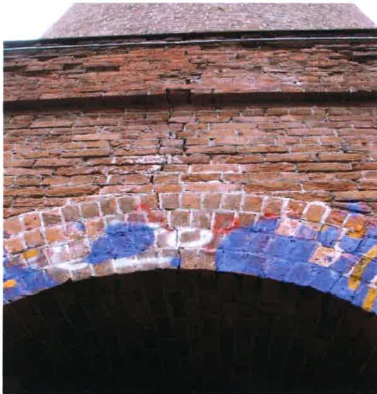
Figure 4 - Close-up of the Vertical Crack
