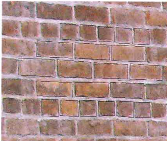
Figure 1 - The brick pattern on the stack wall and the corner building wall is predominantly a 3-layer running bond with stretcher blocks, bounded by single courses of header bricks.
