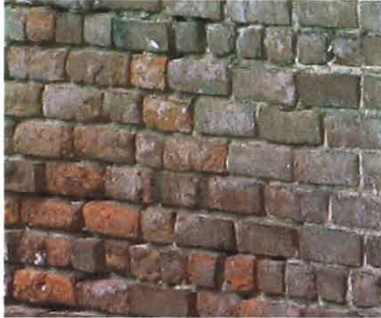
Figure 2 - The only other pattern found on site was for the portion of the partially collapsed flume structure just south of the stack. It shows a common masonry layout with five running bond courses of stretcher blocks laid between single courses of headers
