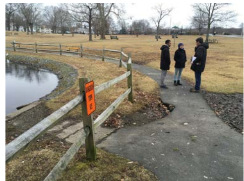
4. Overflow at the edge of Duck Pond.
