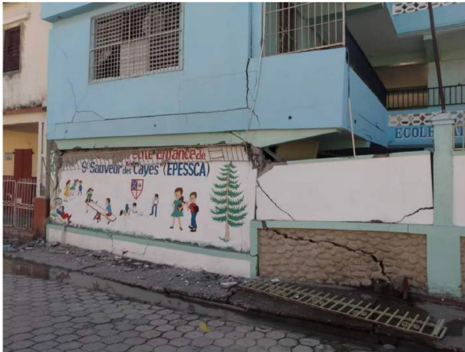
The St. Sauveur des Cayes school in Les Cayes was so damaged beyond repair by the Aug. 14 earthquake and will have to be demolished and rebuilt. Photo: Education Equals Hope
