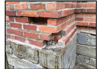
Missing bricks, damaged brick and missing mortar
