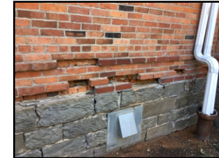
Damaged brick, missing mortar
