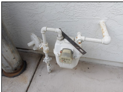
Gas left exterior
