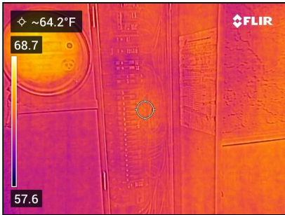
No abnormal heat in electric panel
