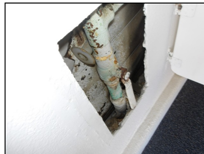
Water in garage
