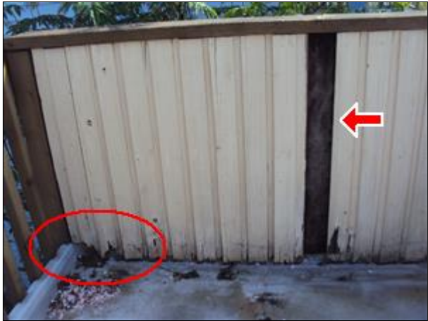
2.0 Picture 3 Missing/Deteriorating Siding
