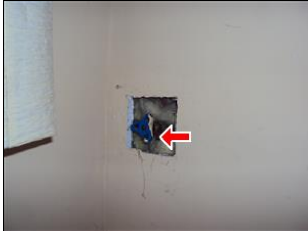
6.3 Picture 1 Main Water Shutoff
