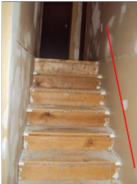
4.3 Picture 1 Missing Handrail
