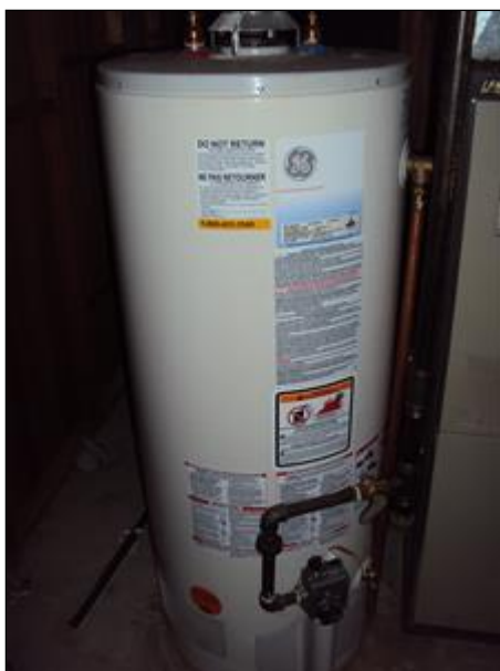
6.2 Picture 1 GE Hot Water Tank
