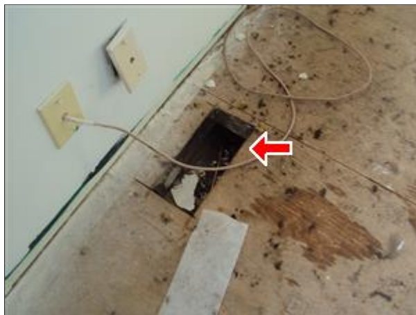
8.3 Picture 1 Missing Vent
