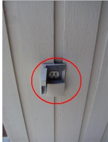
7.3 Picture 4 Non Operational Outlet
