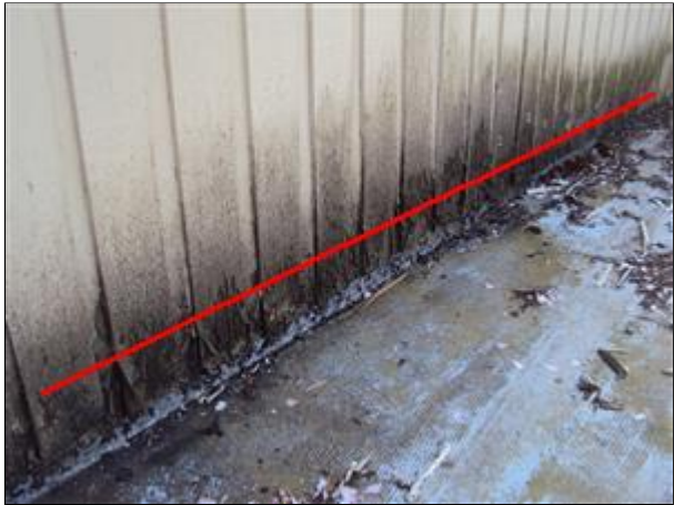
2.0 Picture 1 Deteriorating Siding
