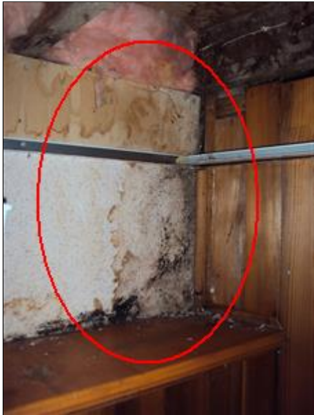
4.1 Picture 3 Water Ingress
