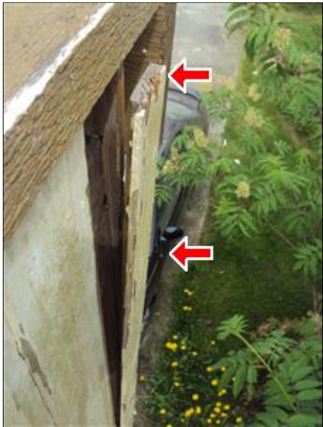
2.0 Picture 4 Loose Siding
