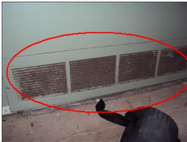
8.3 Picture 2 Clean Ducts
