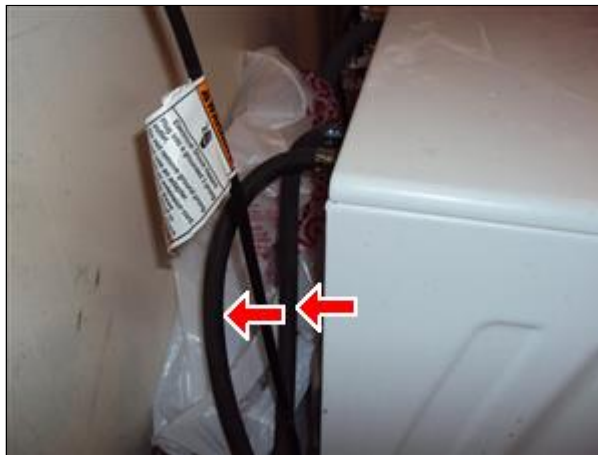
6.1 Picture 2 Washing Machine Hoses
