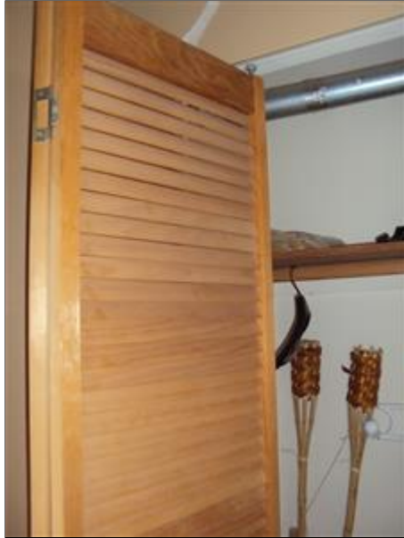
4.5 Picture 1 Non Operational Door
