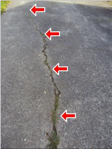
2.3 Picture 7 Settlement Crack
