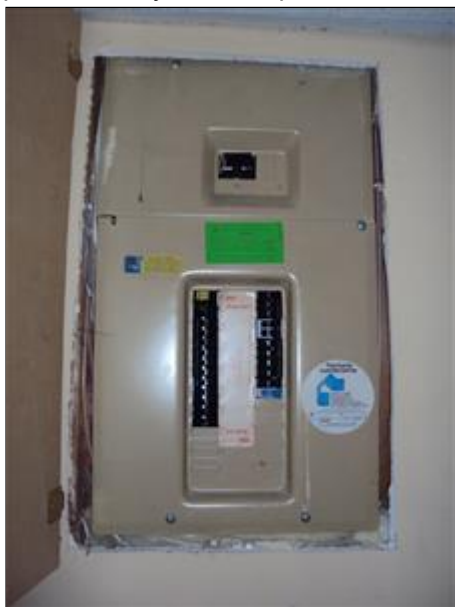
7.6 Picture 1 Electrical Panel
