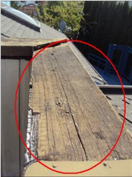
2.0 Picture 2 Deteriorating Trim
