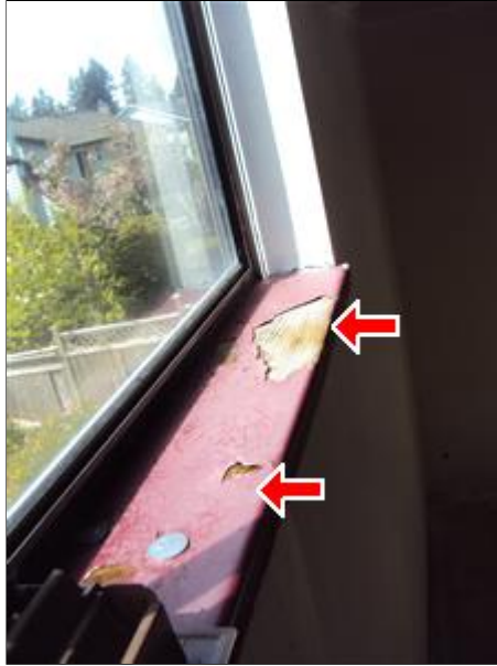
4.6 Picture 1 Deteriorating Paint
