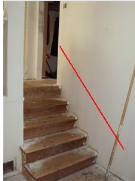
4.3 Picture 2 Missing Handrail
