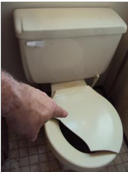
6.1 Picture 1 Loose Toilet
