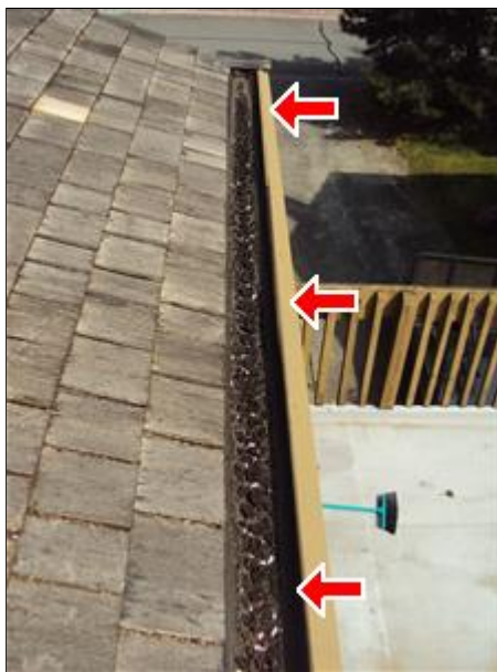
1.3 Picture 1 Clean Gutters
