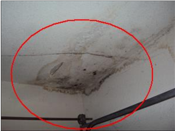
2.3 Picture 3 Water Ingress Garage
