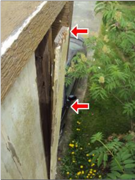
2.0 Picture 4 Loose Siding
