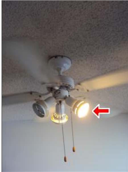
7.3 Picture 7 Loose Fixtures
