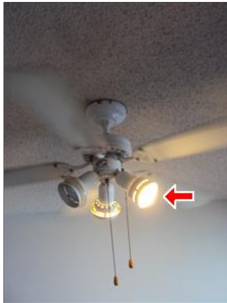
7.3 Picture 7 Loose Fixtures
