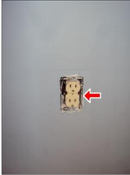
7.3 Picture 1 Missing Cover Plate
