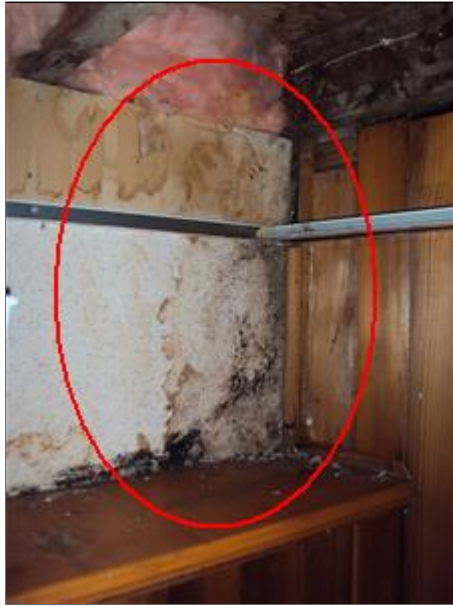
4.1 Picture 3 Water Ingress
