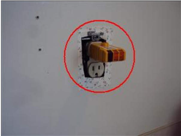
7.3 Picture 3 Non Operational Outlet
