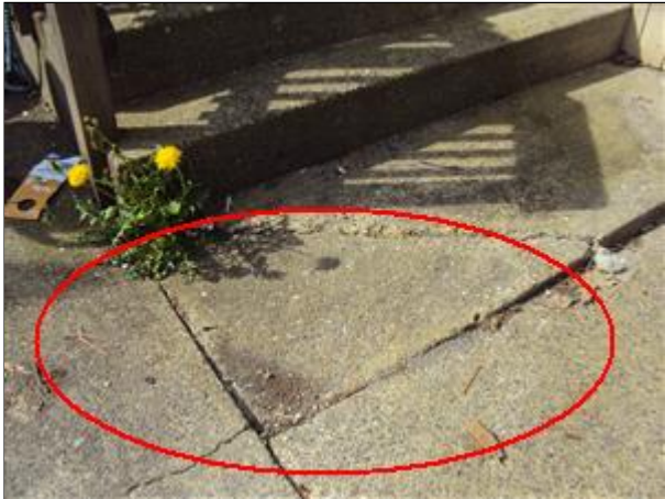
2.3 Picture 6 Settlement Crack
