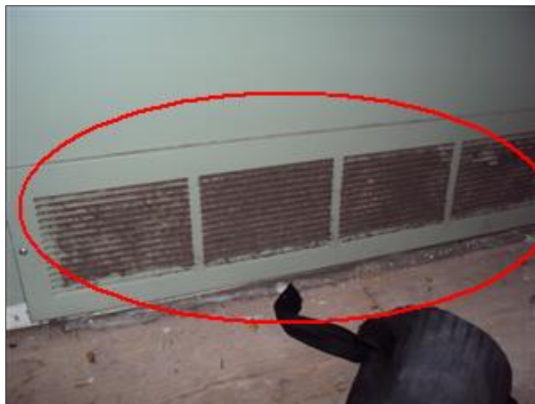
8.3 Picture 2 Clean Ducts
