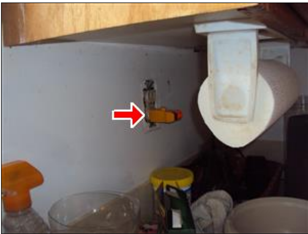
7.3 Picture 6 Not GFCI Protected
