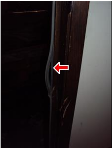
3.4 Picture 2 Failed Door Seal
