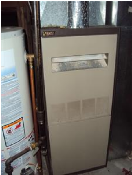
8.0 Picture 1 Lennox Furnace
