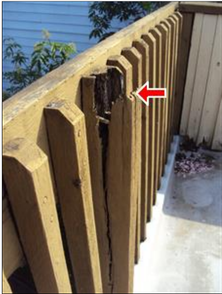
2.3 Picture 1 Rotting Support Post
