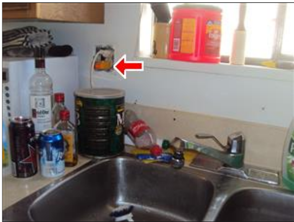
7.3 Picture 5 Not GFCI Protected
