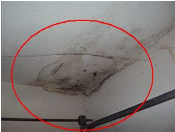
2.3 Picture 3 Water Ingress Garage
