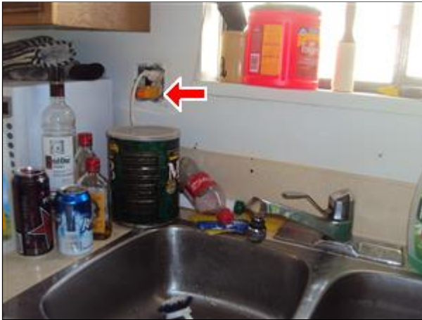
7.3 Picture 5 Not GFCI Protected
