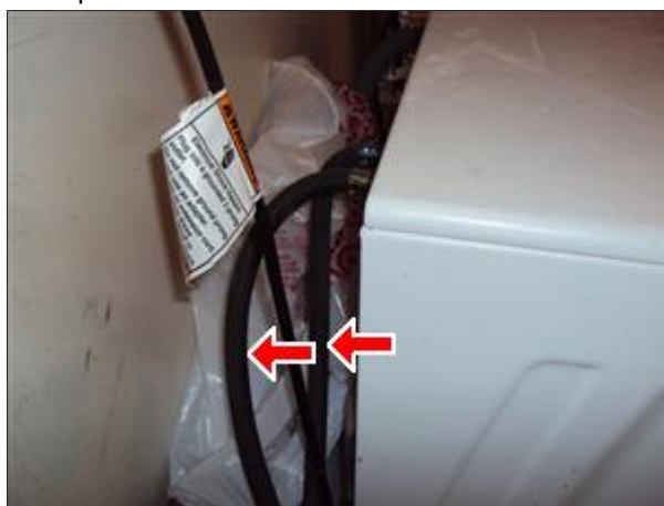
6.1 Picture 2 Washing Machine Hoses
