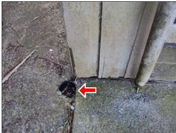
2.4 Picture 3 Failed Perimeter Drain
