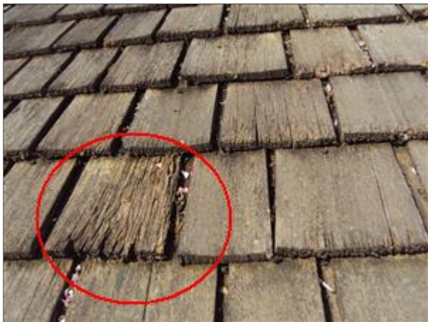
1.0 Picture 1 Shingle Deterioration
