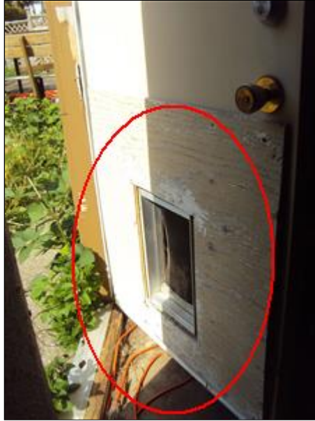
2.1 Picture 3 Deteriorating Door
