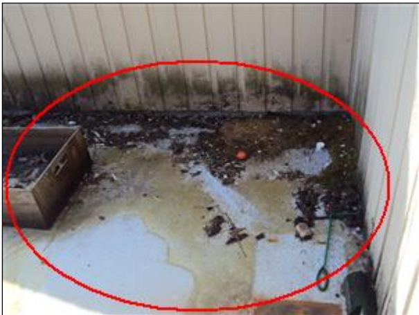
2.3 Picture 5 Balcony Deterioration
