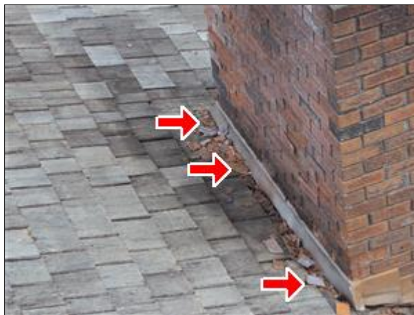
1.2 Picture 1 Brick Debris Chimney
