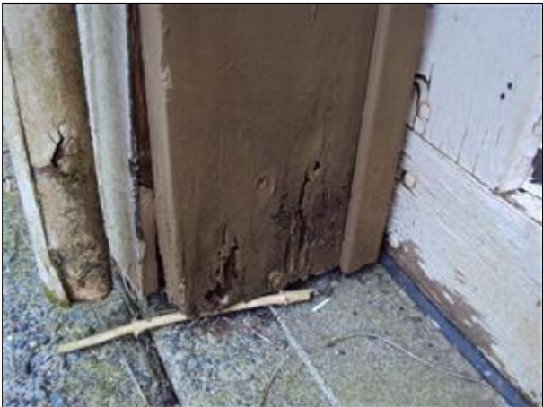
2.0 Picture 5 Deterioration Trim
