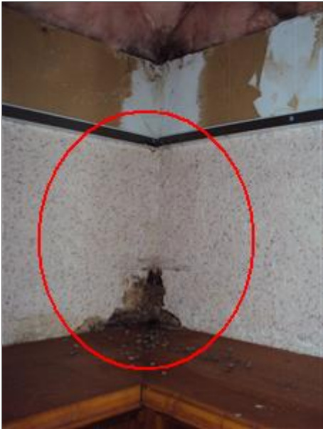
4.1 Picture 4 Water Ingress
