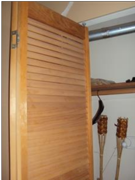
4.5 Picture 1 Non Operational Door
