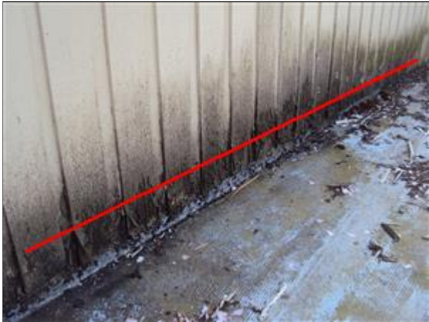
2.0 Picture 1 Deteriorating Siding
