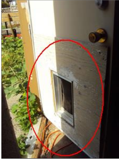
2.1 Picture 3 Deteriorating Door
