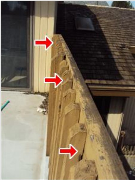
2.3 Picture 2 Loose Railing
