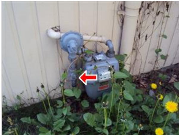
6.5 Picture 1 Main Fuel Shutoff
