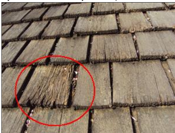
1.0 Picture 1 Shingle Deterioration
