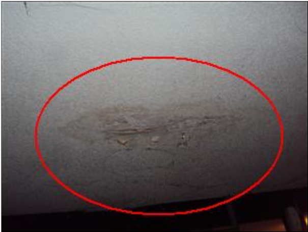
2.3 Picture 4 Water Ingress Garage
