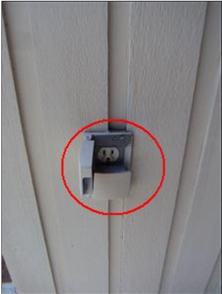
7.3 Picture 4 Non Operational Outlet
