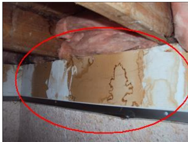
4.1 Picture 5 Water Staining
