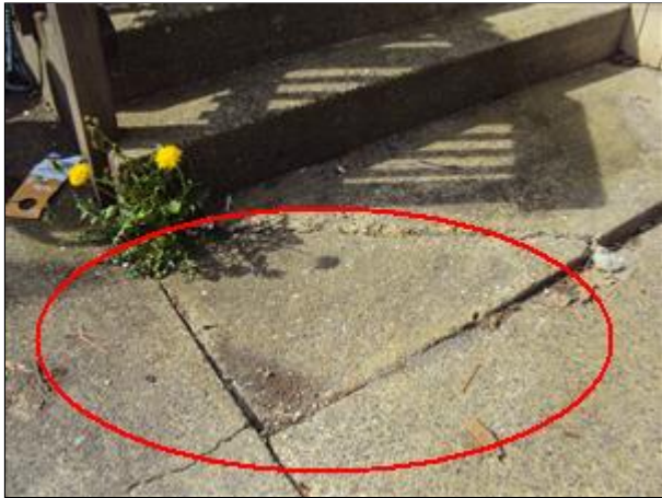
2.3 Picture 6 Settlement Crack
