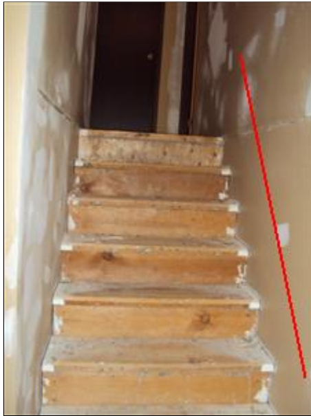
4.3 Picture 1 Missing Handrail
