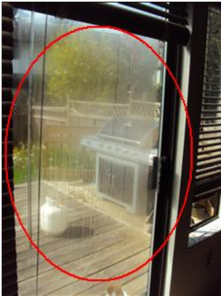
2.2 Picture 1 Failed Sliding Door Seal
