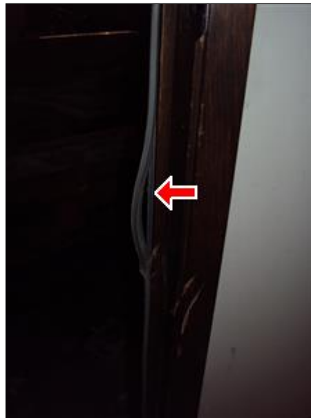
3.4 Picture 2 Failed Door Seal
