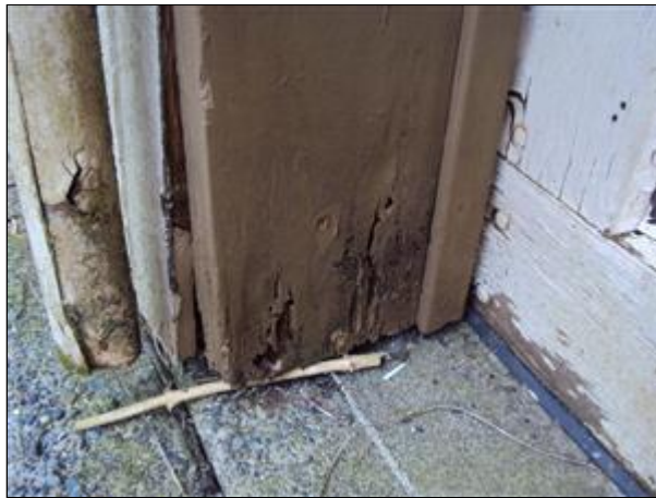
2.0 Picture 5 Deterioration Trim
