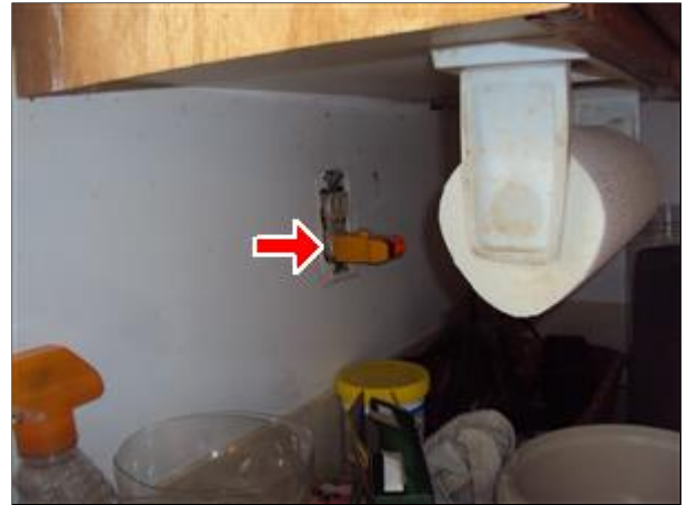
7.3 Picture 6 Not GFCI Protected
