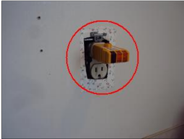
7.3 Picture 3 Non Operational Outlet
