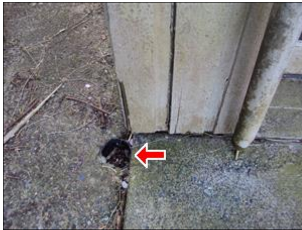
2.4 Picture 3 Failed Perimeter Drain
