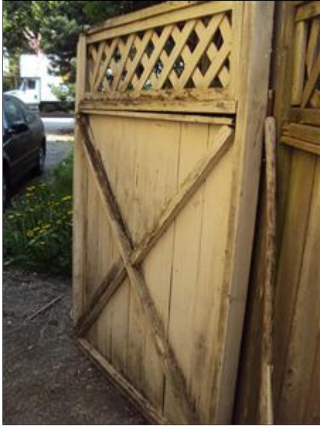
2.6 Picture 1 Non Operational Gate
