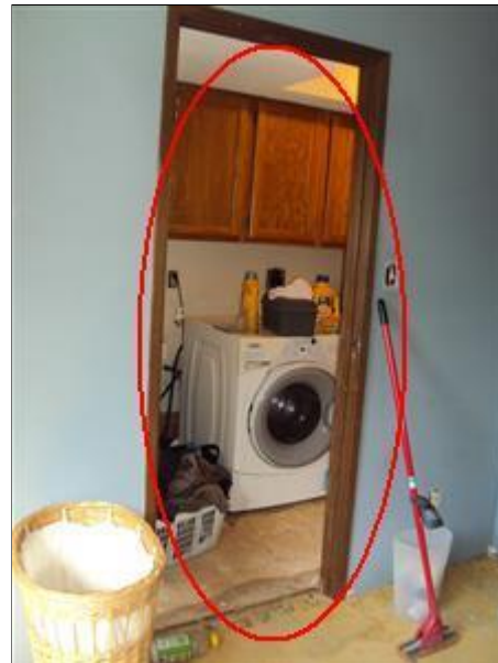
4.5 Picture 2 Missing Door
