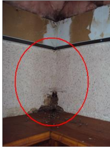
4.1 Picture 4 Water Ingress
