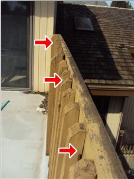
2.3 Picture 2 Loose Railing
