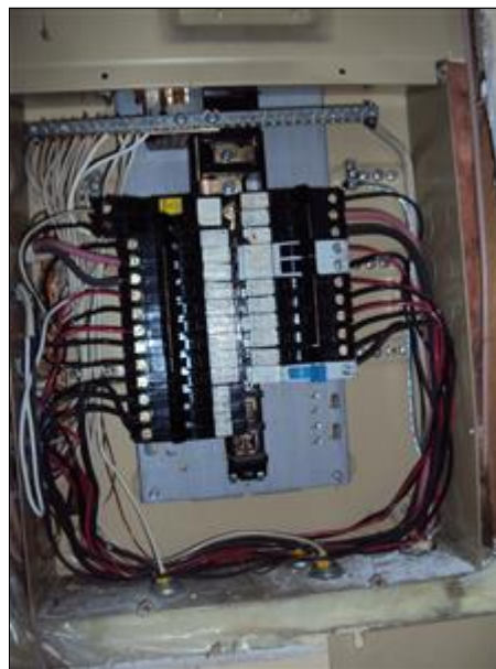
7.6 Picture 2 Branch Wiring
