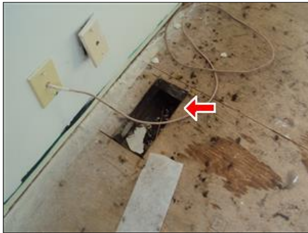
8.3 Picture 1 Missing Vent
