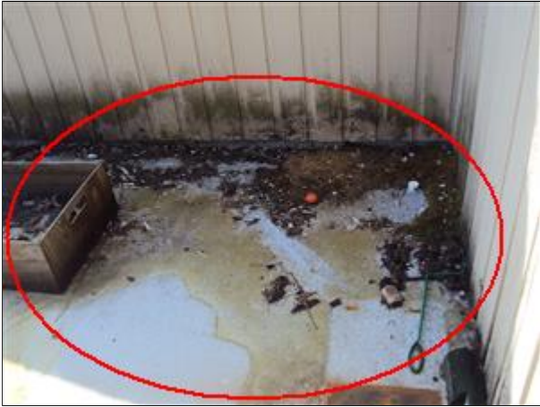
2.3 Picture 5 Balcony Deterioration
