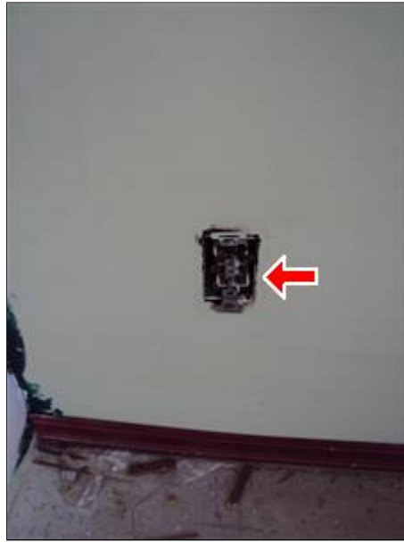
7.3 Picture 2 Exposed Outlet
