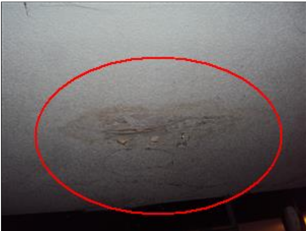
2.3 Picture 4 Water Ingress Garage
