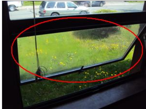
2.2 Picture 2 Failed Window Seal
