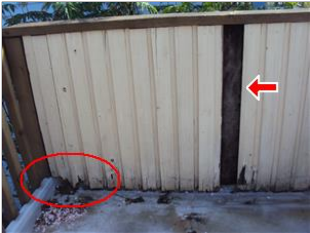
2.0 Picture 3 Missing/Deteriorating Siding
