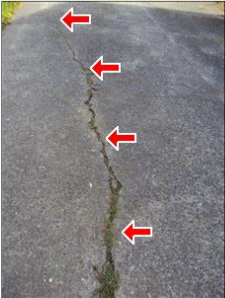
2.3 Picture 7 Settlement Crack
