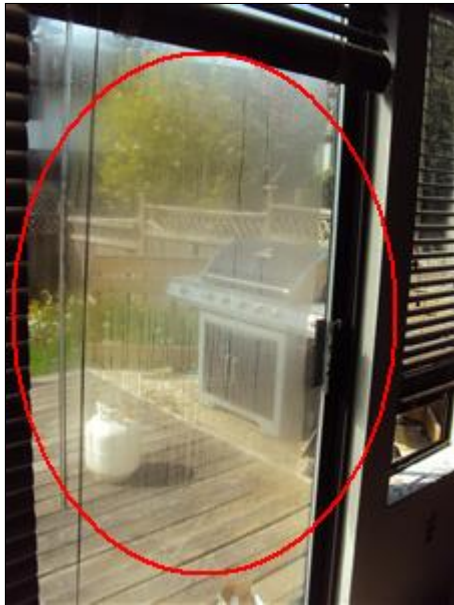
2.2 Picture 1 Failed Sliding Door Seal
