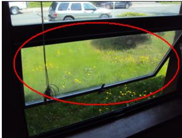
2.2 Picture 2 Failed Window Seal
