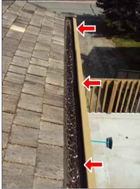
1.3 Picture 1 Clean Gutters
