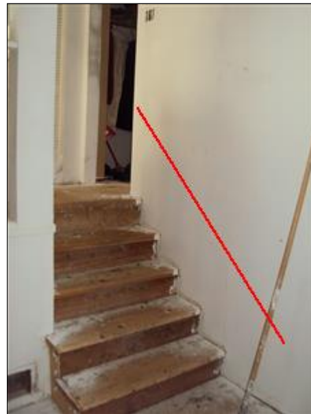
4.3 Picture 2 Missing Handrail
