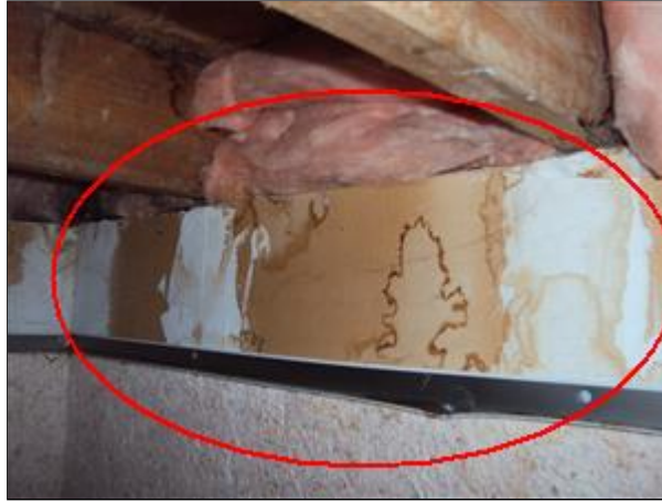
4.1 Picture 5 Water Staining
