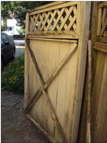
2.6 Picture 1 Non Operational Gate
