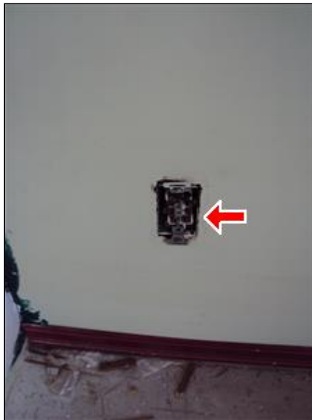
7.3 Picture 2 Exposed Outlet
