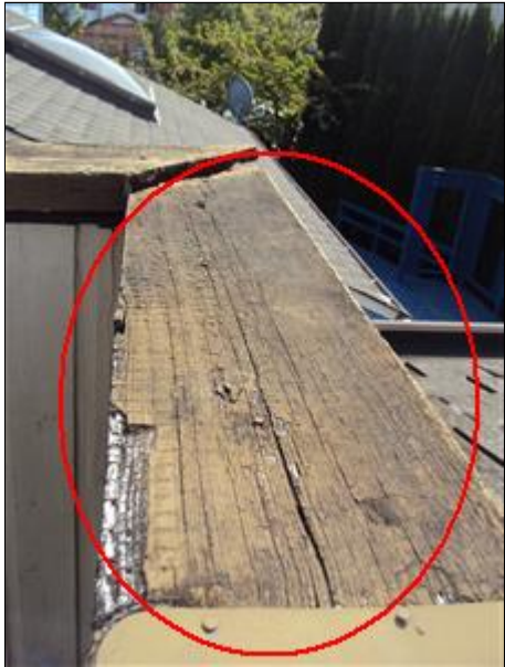
2.0 Picture 2 Deteriorting Trim
