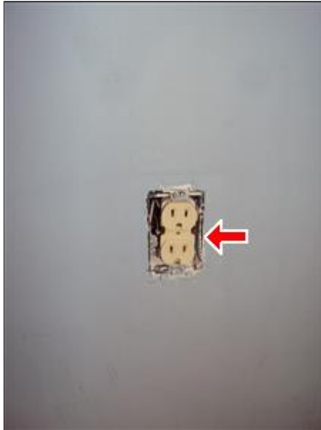
7.3 Picture 1 Missing Cover Plate
