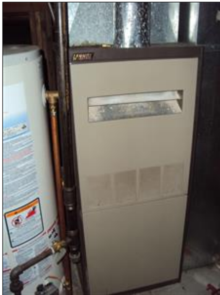
8.0 Picture 1 Lennox Furnace
