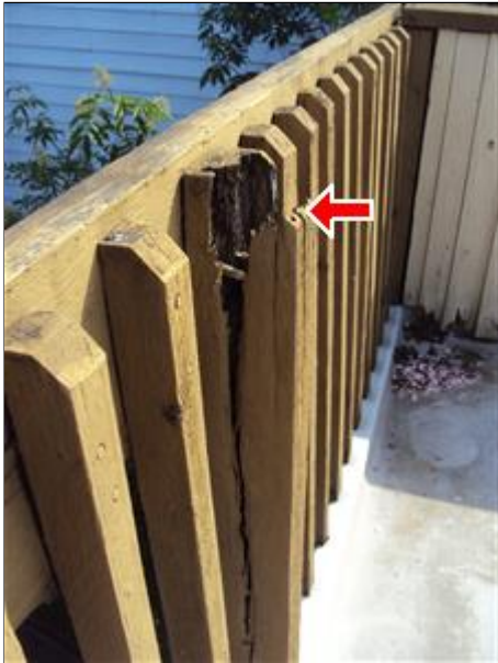
2.3 Picture 1 Rotting Support Post
