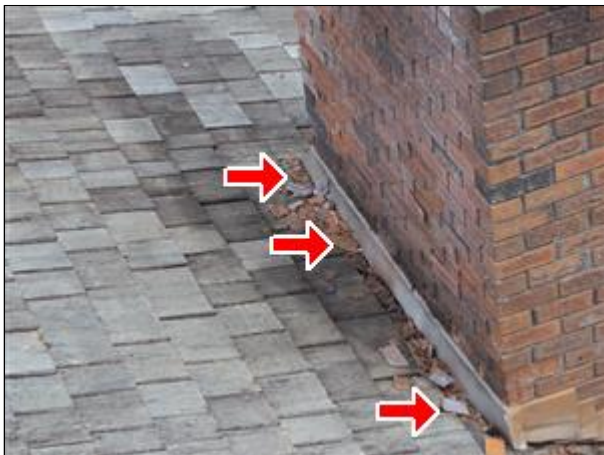
1.2 Picture 1 Brick Debris Chimney
