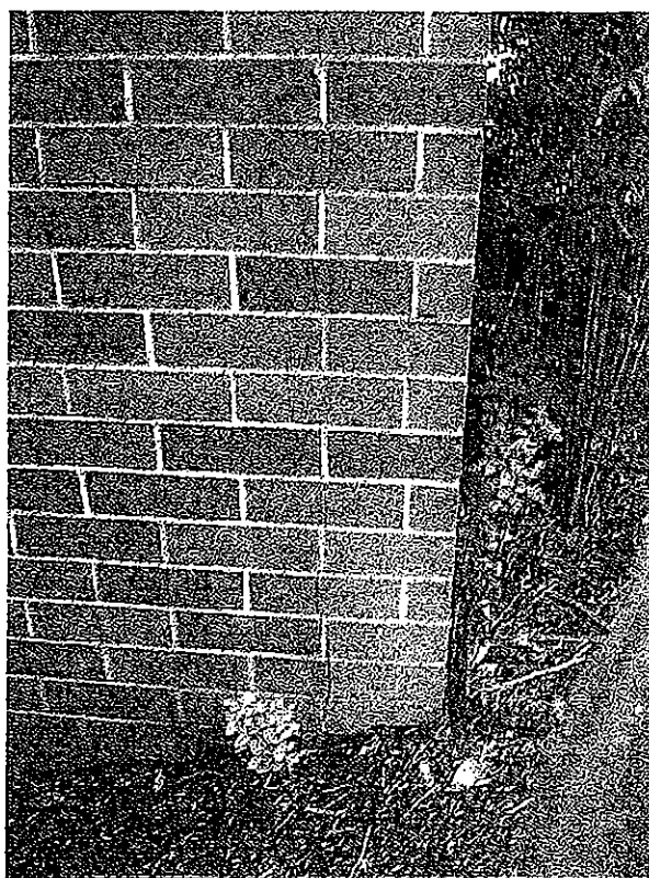
Photo 6: Stairwell Masonry Cracks
