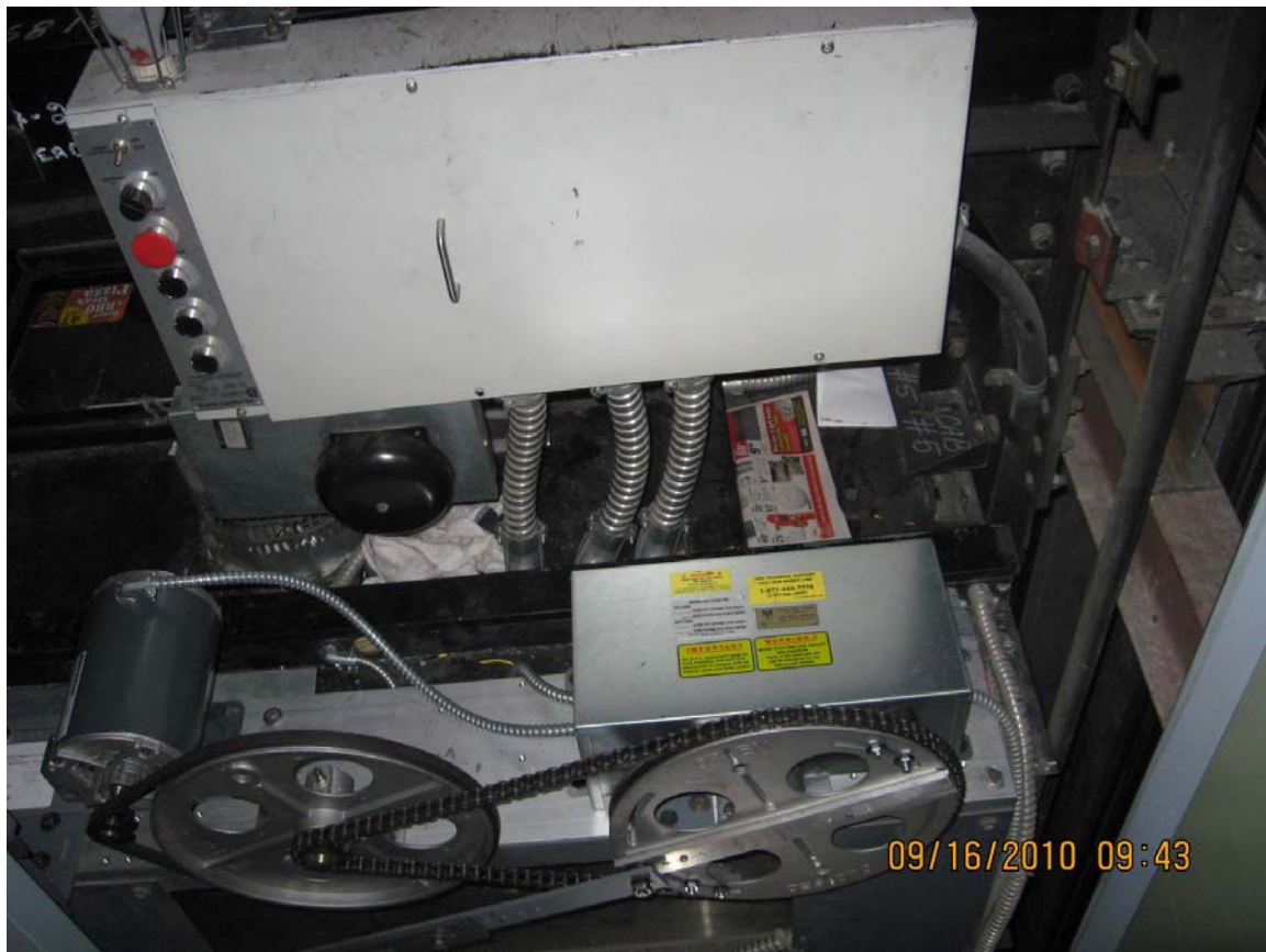
Photo 7 – Elevator Car Top
