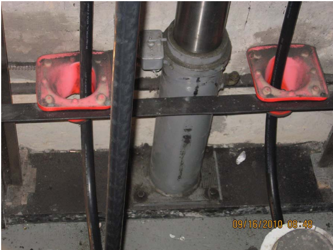
Photo 3 – Elevator Pit - Note pylon used for compensation guides
