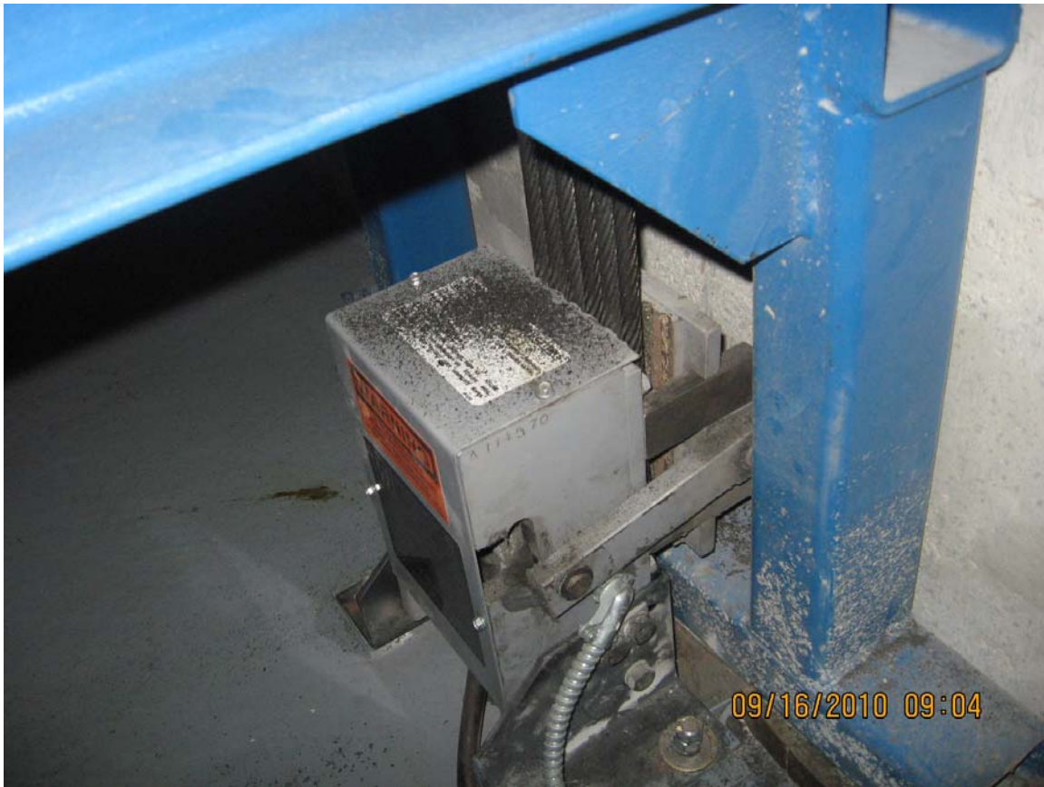
Photo 9 – Auxiliary Brake - Rope Gripper
