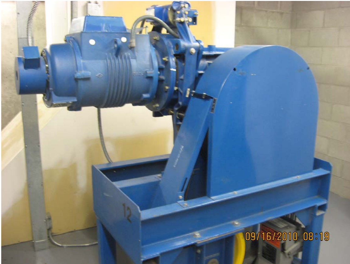
Photo 11 – Elevator Hoist Machine
