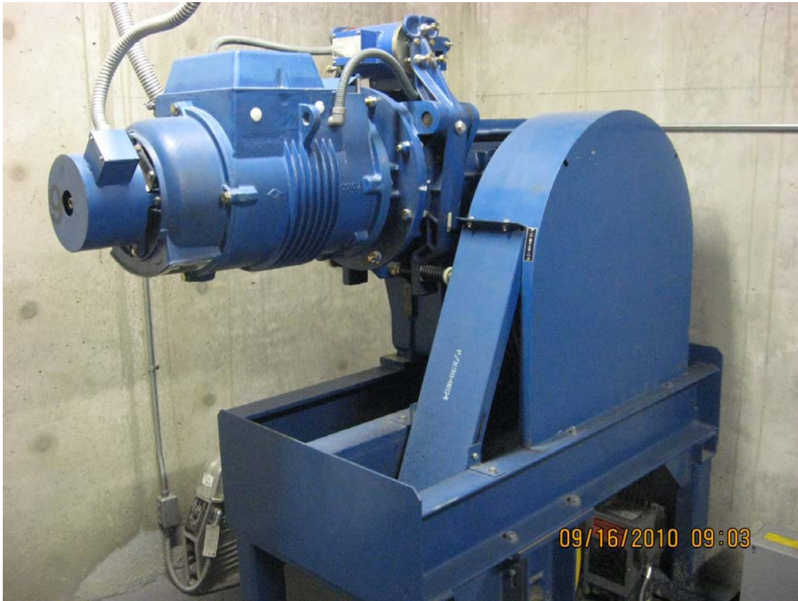
Photo 8 – Elevator Hoist Machine
