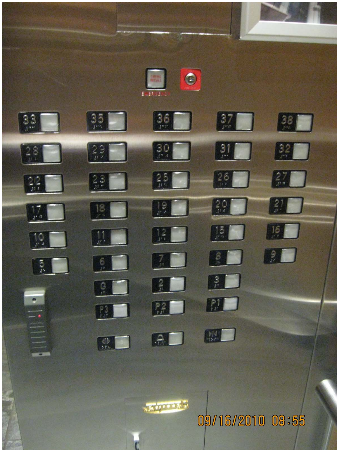
Photo 4 – Elevator Interior - Car Operating Panel
