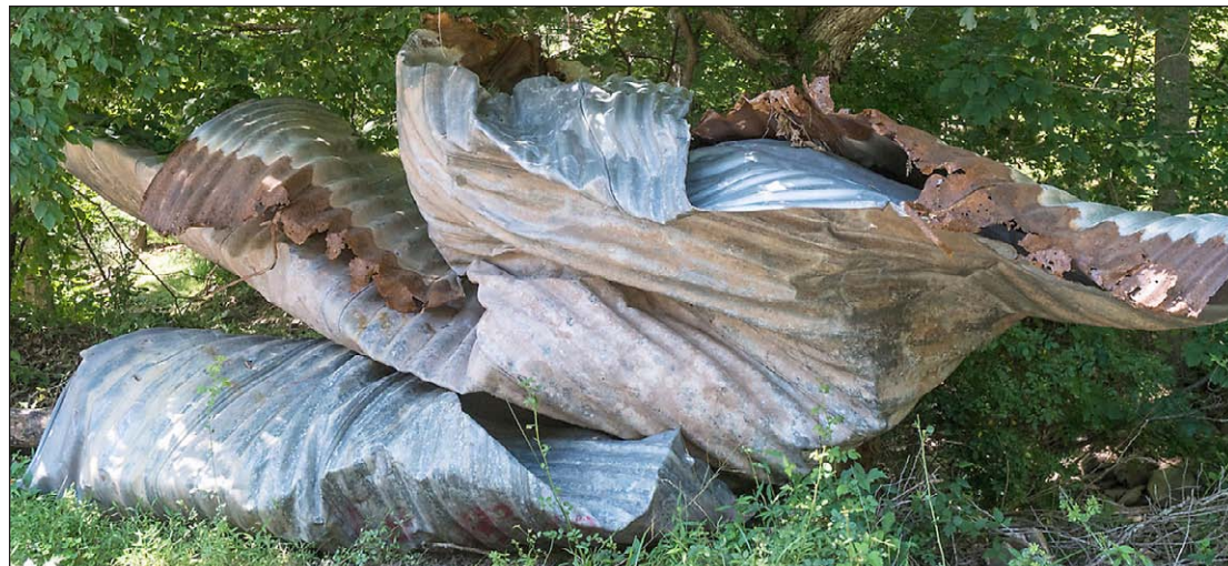
Rampaging waters from the storms in late June left this culvert twisted like a pretzel, and closed Perry Whetzel Road where it intersects Cullers Run for several days.
