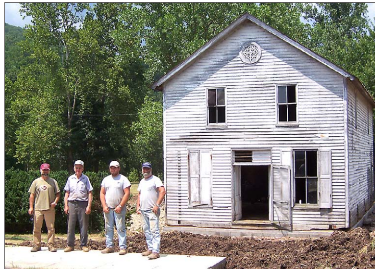
Earl Miller & Sons were happy with a job well done after the store was set on the foundation.
