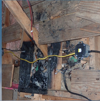
Lightning struck this house and started a small fire.
