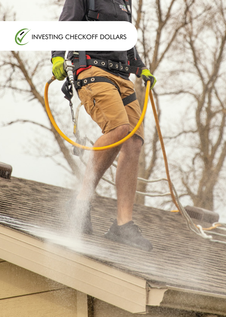
When considering options to maximize the longevity of a rental property, Bonnie and Craig Dybedahl looked to soy. Soy-based roof preservative by Roof Maxx was applied to a home near Colton, S.D.
